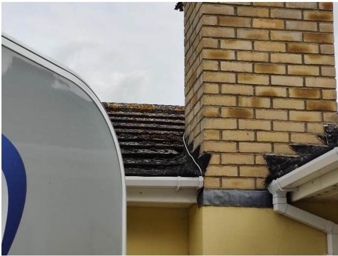
Photo 13 Gap under tile adjacent to the chimney on the northwest elevation
