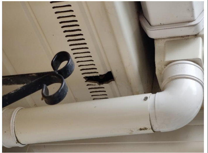
Photo 14 Hole in soffit on the southeast elevation, adjacent to the conservatory
