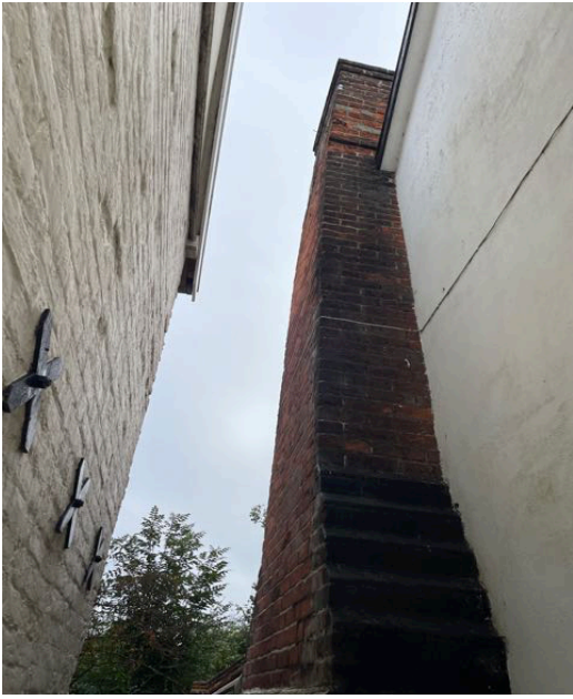
HIGH LEVEL VIEW of CHIMNEY STACK of 21 and SIDE WALL (EAST) of 23
