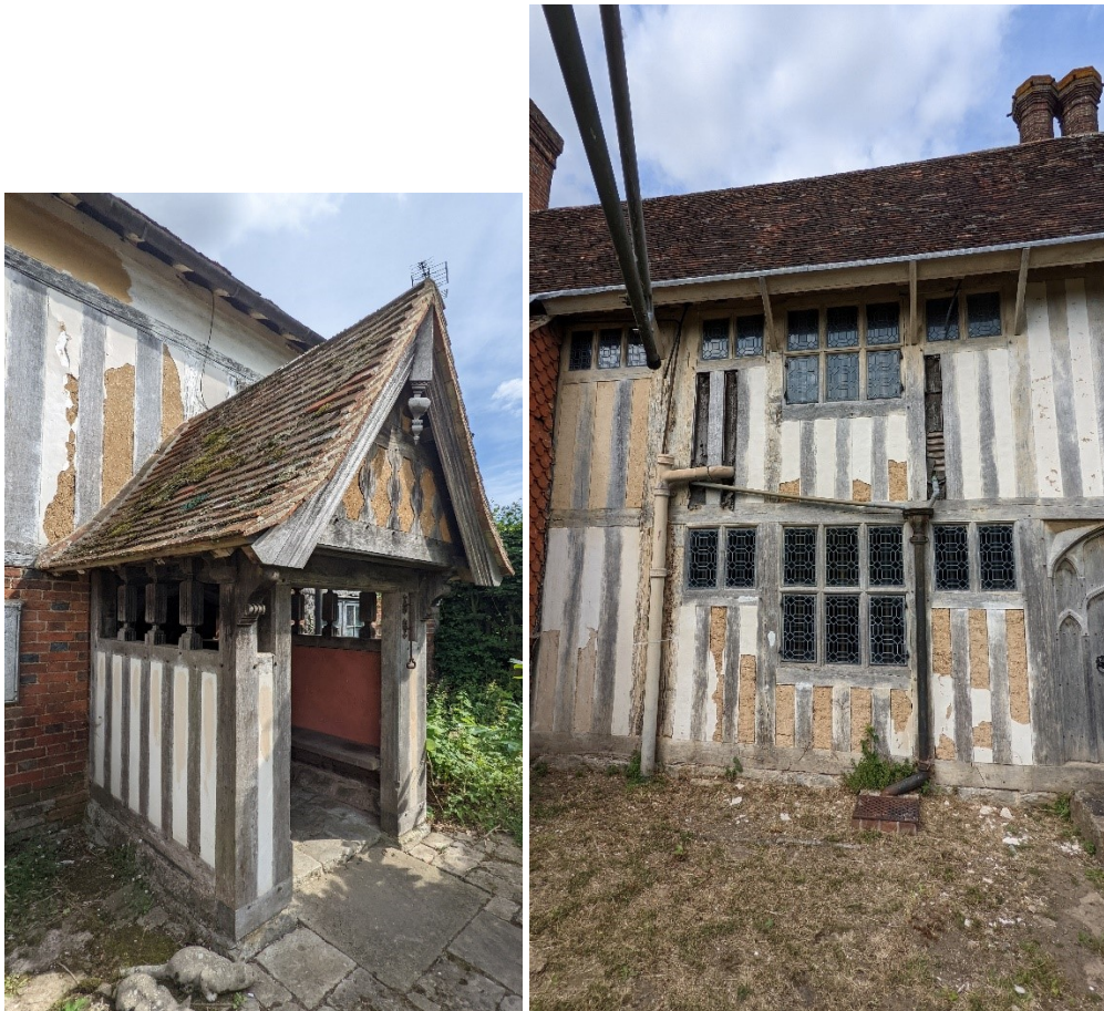
Fig. 1 (left) Part of west elevation with modern porch, fig.2 (right) part of the south elevation, showing extensive damage to the late C20 render infill.
