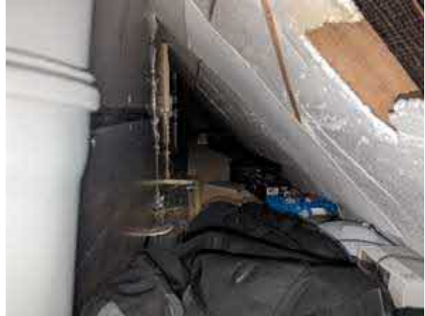
Photo 4. Showing the roof void at the eaves on the front of the building
