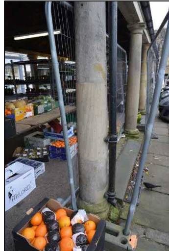
COLUMN Original Heavily repaired recent middle section NHL plastic repair to small hole
