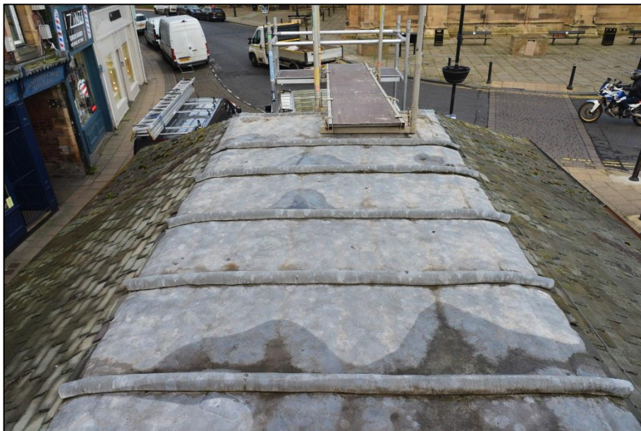
The standing water seem to coincide with the locations of the damaged and deflecting trusses.
