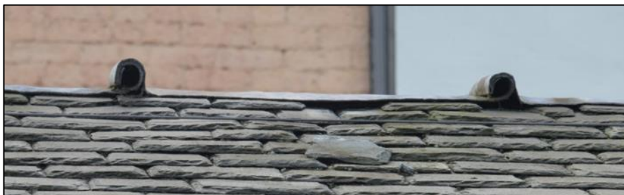
The open lead rolls will have been formed around a heavy sisal rope.
