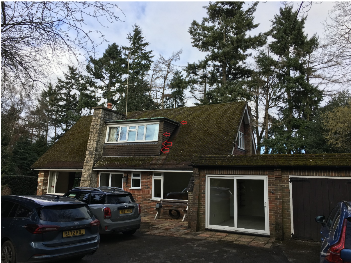
Figure 5. South and east elevations of bungalow looking north. Red arrow indicates opening into soffit.
