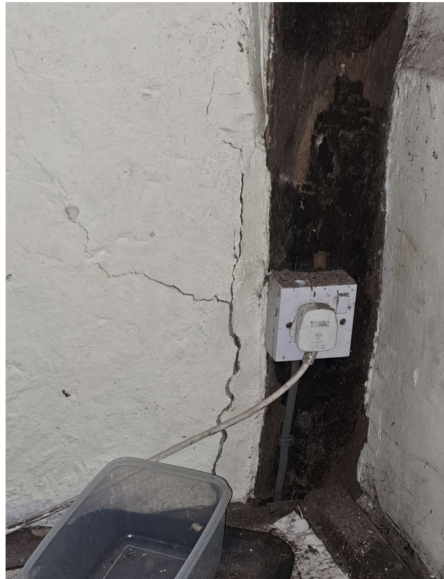
Figure 10 Cracking in North-West Corner
