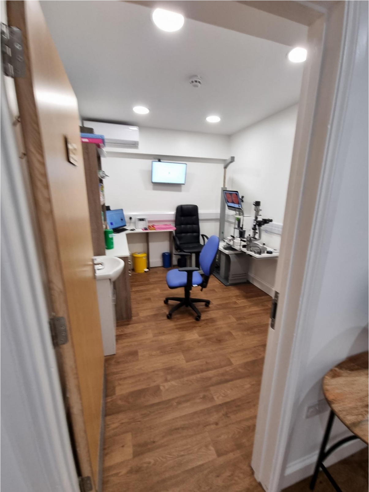
Figure 3 – individual treatment rooms, with air con units at high level.
