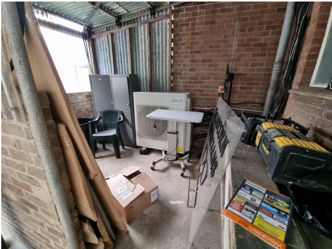
Figure 7 – rear elevation with pipework for air handling unit and intact.
