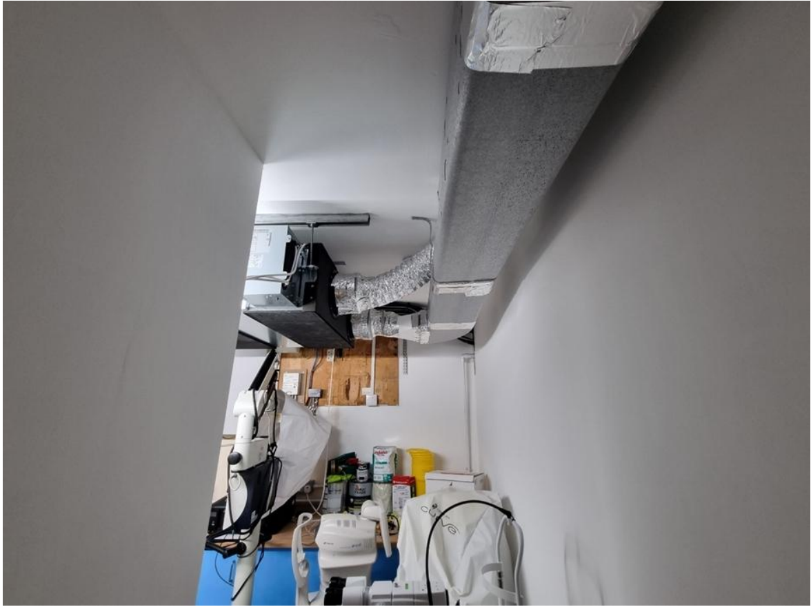
Figure 6 – pipework for air intake to supply the rear rooms.
