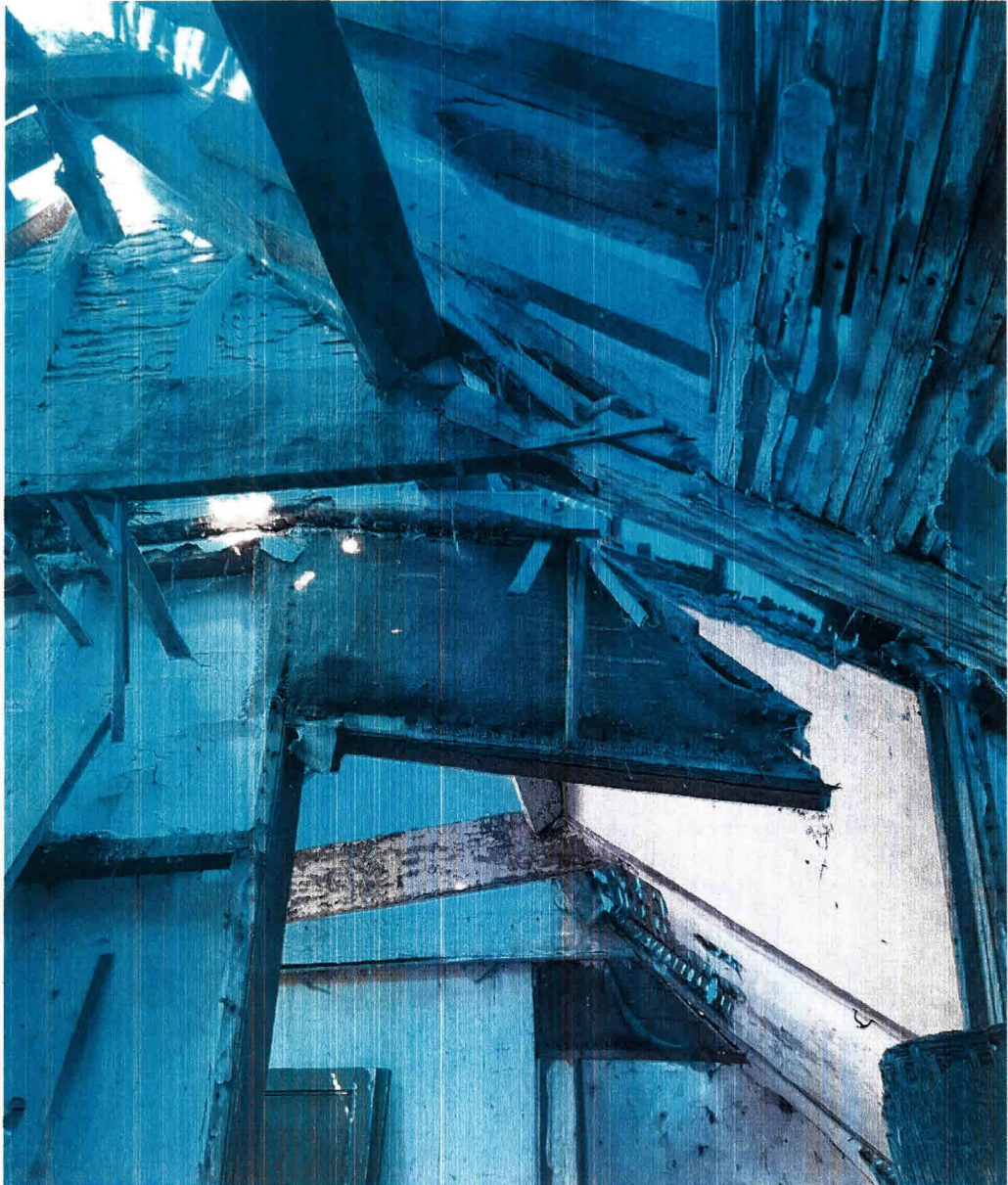
Structural Failure of Principal Rafter (Note – Mortice for collar and elongated birds' mouth over clasped purlin, plus further failing principle frame beyond)
