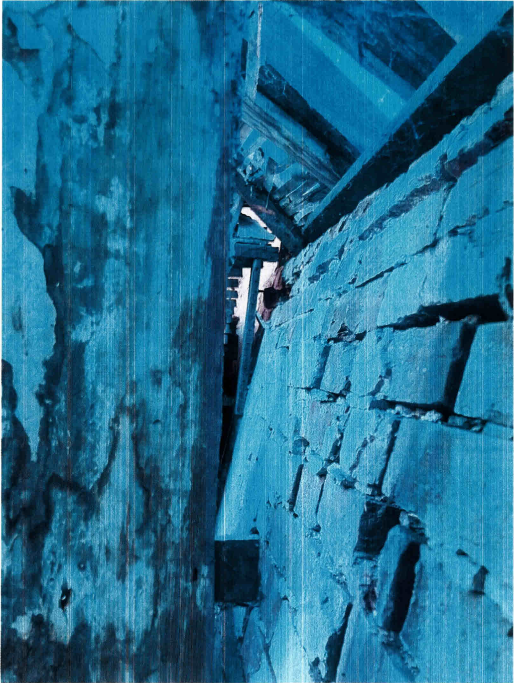
Extent of lateral movement (spread) of top of wall and wall plate
