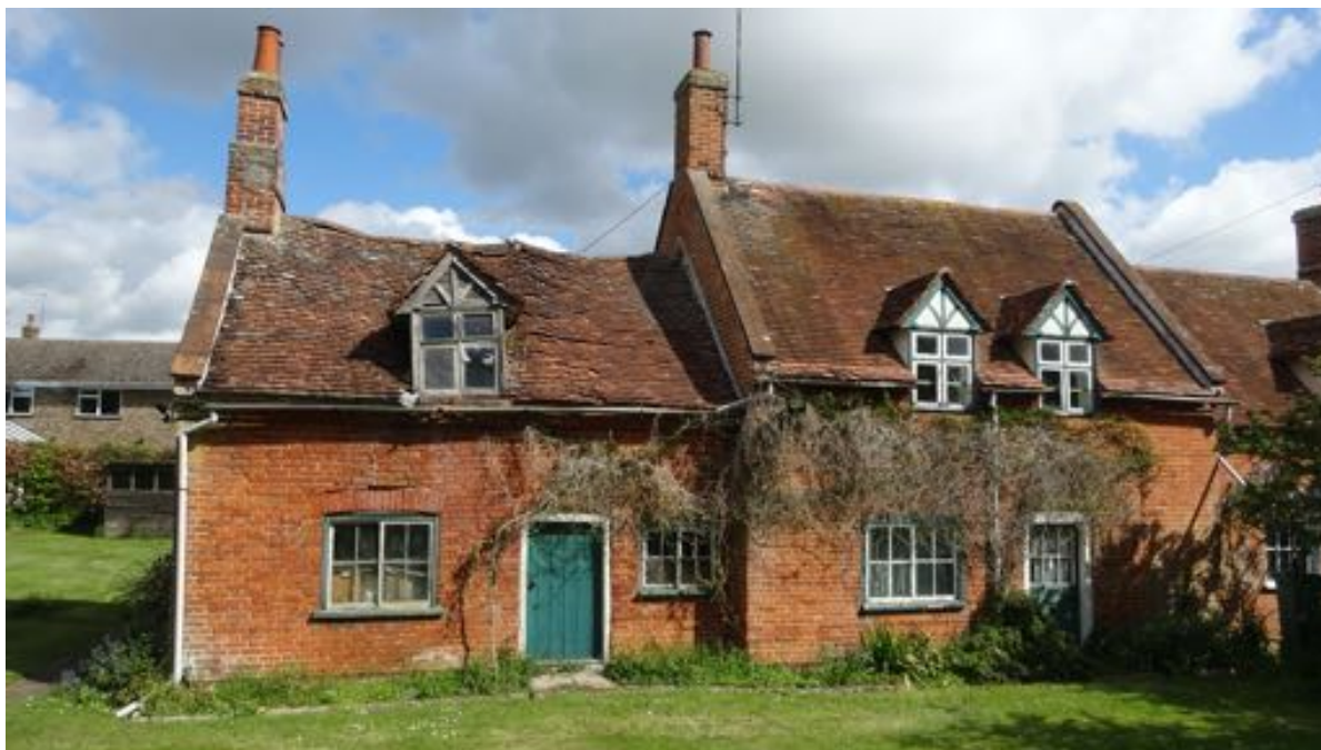
Image 2. South (front) elevation (May 2021). Image of the principle elevation showing the 2 no. structures visible with 23 having a higher ridge and is still habitable. No. 24 is derelict and is not habitable in its current form.
