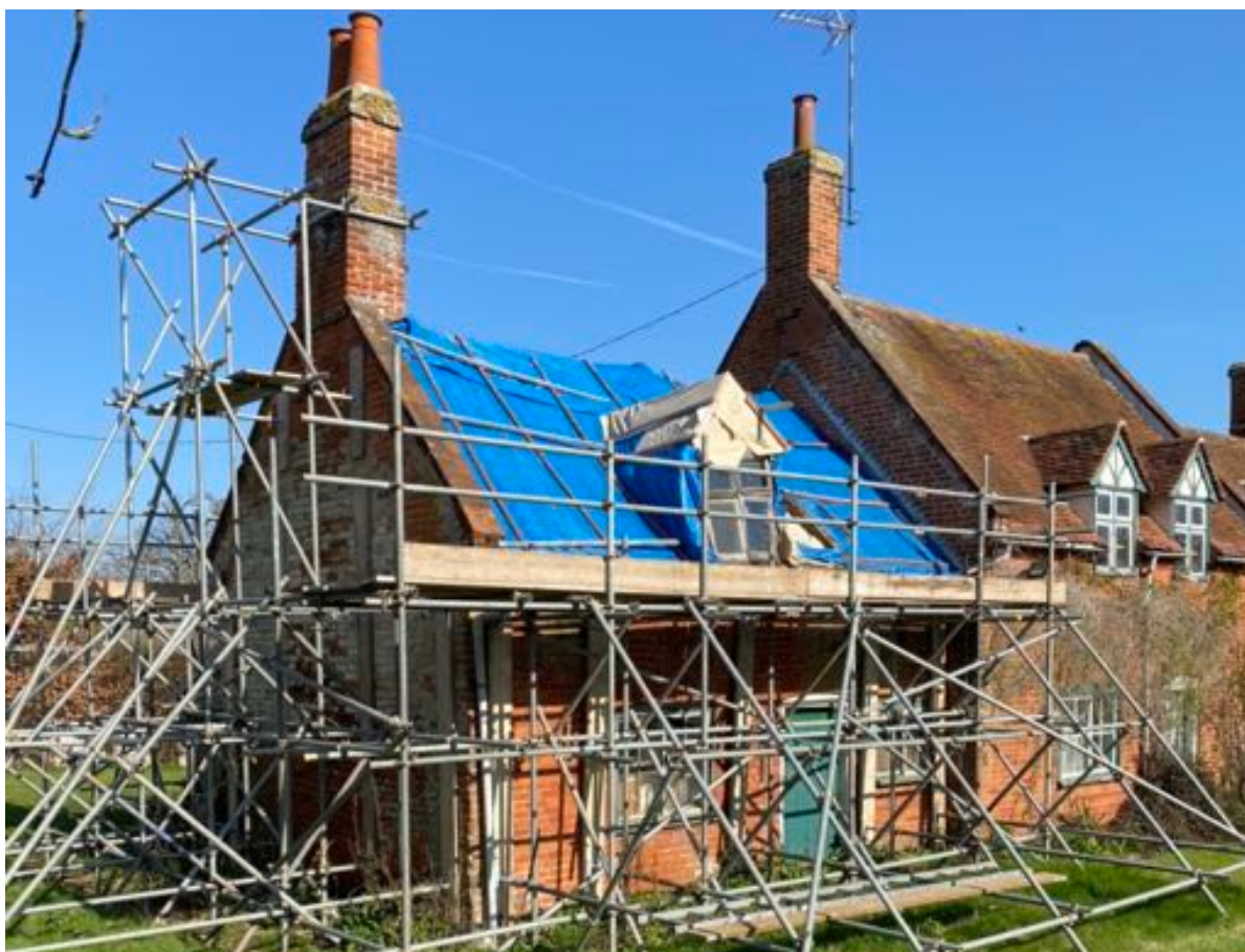
Image 3. South (Front) Elevation (March 2022). This image shows No. 24 is in a significant state of disrepair and will require a large element of reconstruction, The building has been 'propped' to avoid total collapse however, the built structure continues to deteriorate. This is clearly visible there the lead flashing meets no. 23 illustrating how much the roof has 'dropped'.
