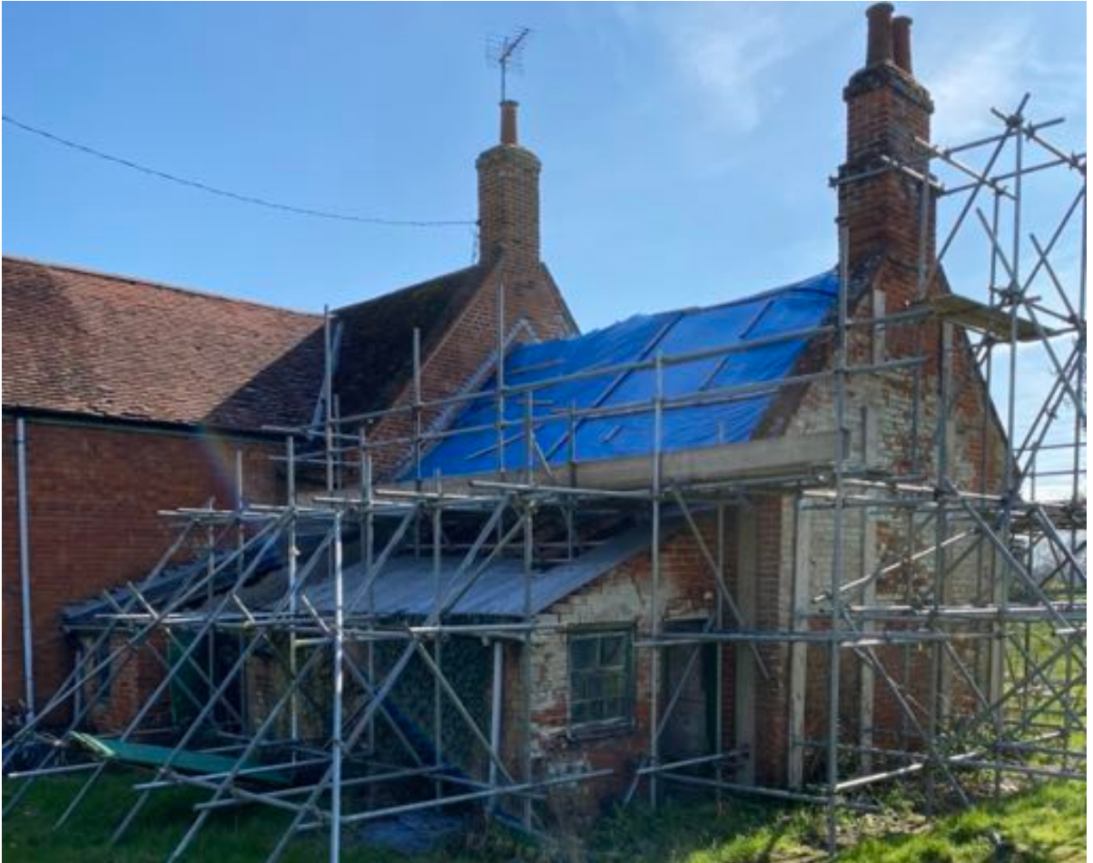
Image 5. West Elevation (March 2022). This image shows both 23 & 24 with the single storey lean-to additional and the two storey extension to the rear of no. 24. As with image 3, this clearly shows the significant deterioration over the past 10 months
