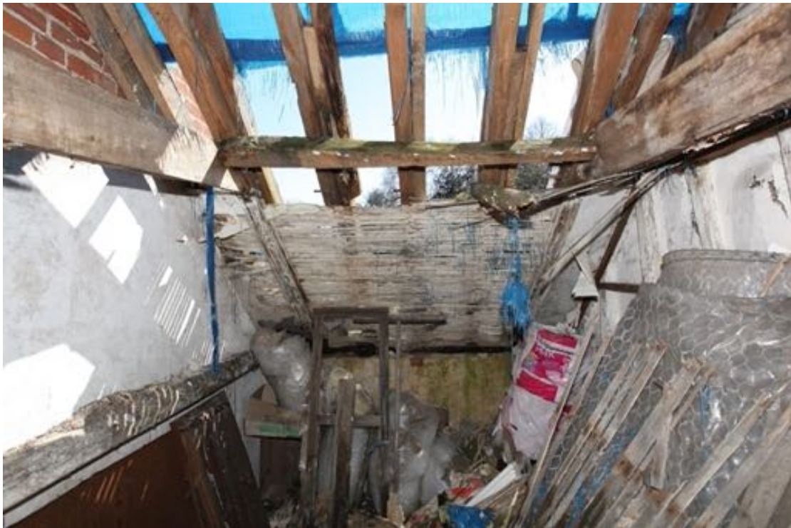
Illus. 28. The narrow stair landing of no. 24 as seen from the north (F2), showing the structure's clasped-purlin roof with pegged collars and narrow-sectioned purlins. The remains of a lath-and-plaster ceiling that extended to the collars survive on the rafters.
