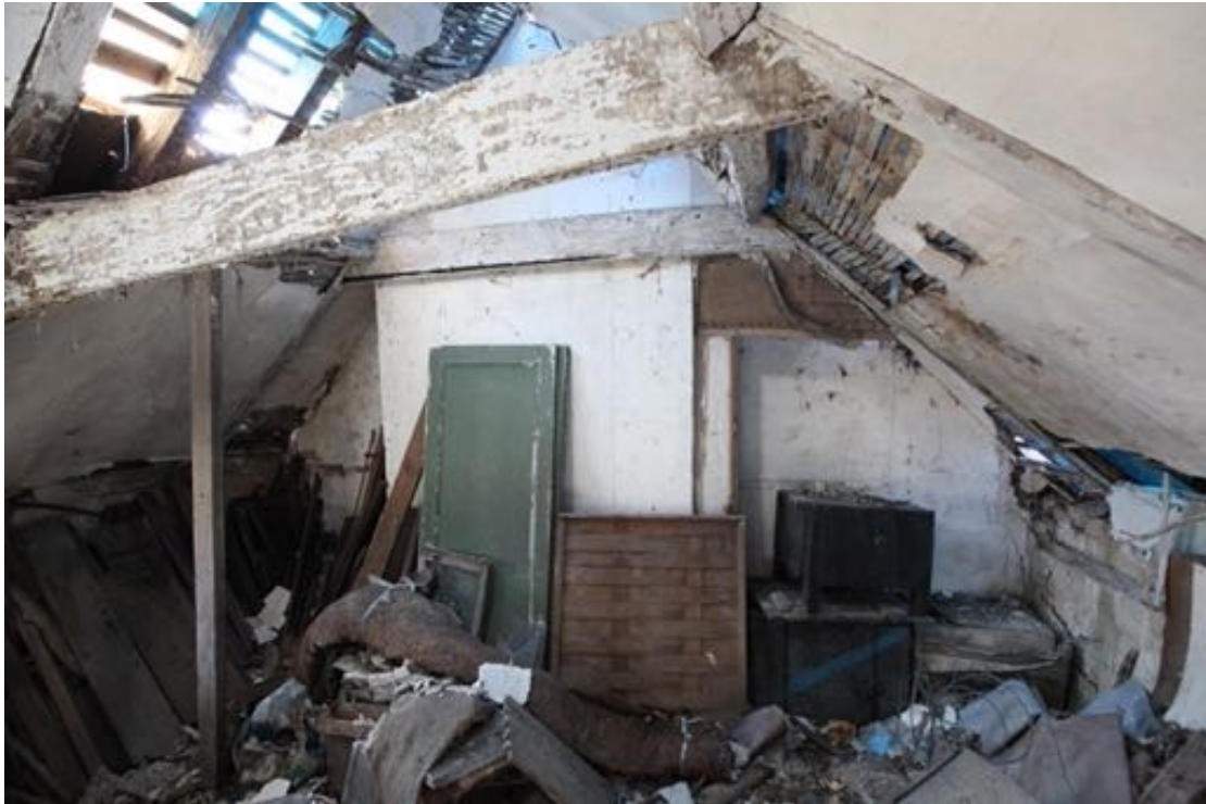
Illus. 33. The first-floor bedroom at no. 24 from the east showing the rendered chimney breast against its western gable (F1).
