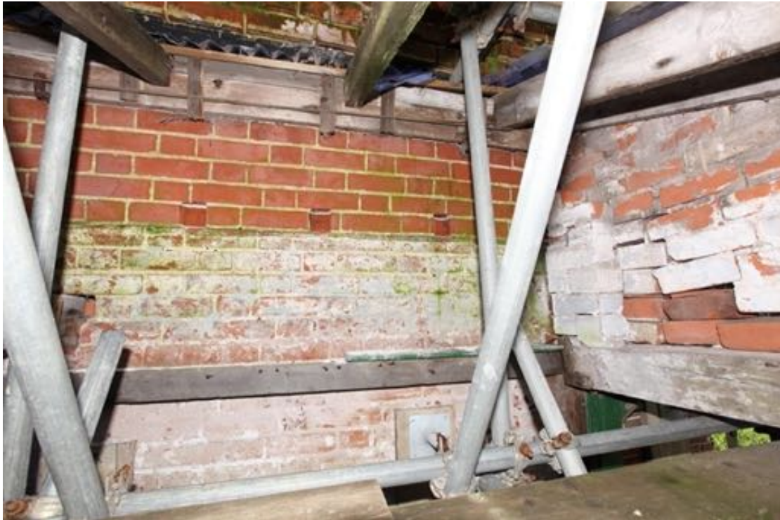
Illus. 13. The rear wall of no. 24 from its rear lean-to (G3) showing the windowless brickwork demonstrating that a lean-to existed in this position from the outset. The present western brick gable of the lean-to on the right is a later addition that is not keyed to the wall so the existing structure probably replaced a timber-framed predecessor.
