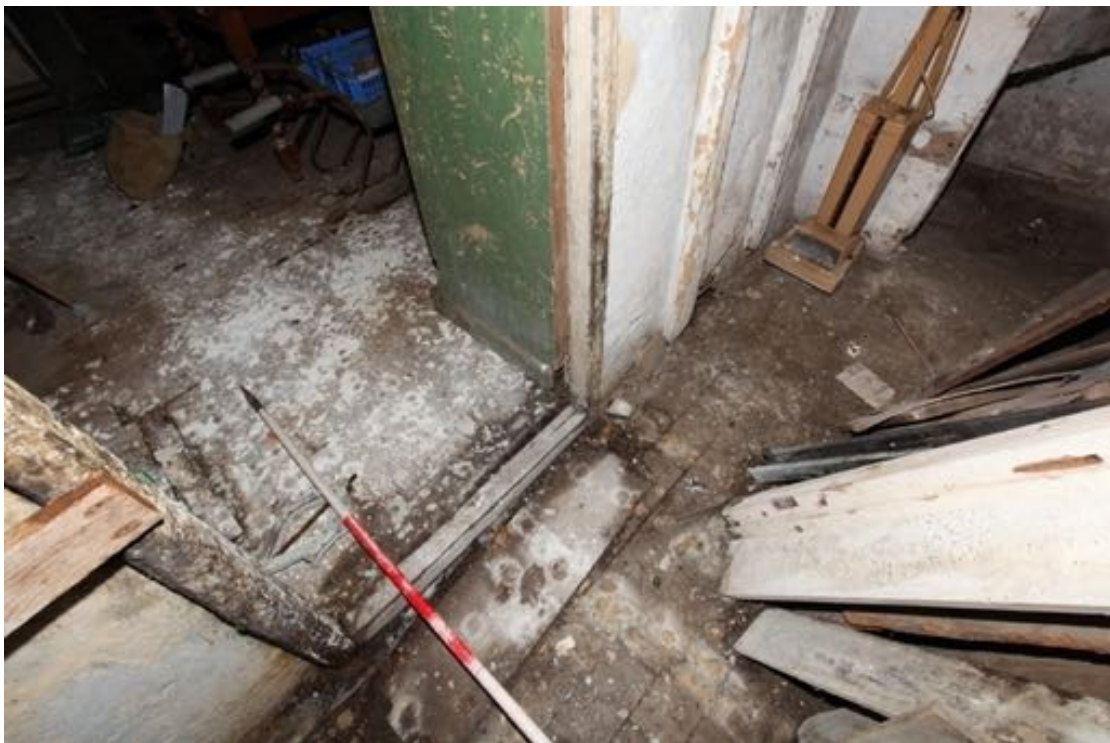
Illus. 26. A detail of the 19 th century gault floor bricks in the storage area in front of the stair in no. 24 (G2), as seen from the south.
