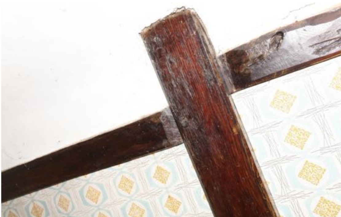
Illus. 50. A detail of the staggered butt-purlins with chamfered ends and pegged joints in the southern elevation of the eastern bedroom in no. 23 (F4). A second tier of matching purlins is hidden above the ceiling. The use of pine timber and the butt-purlin structure is typical of the early- to mid-19 th century.
