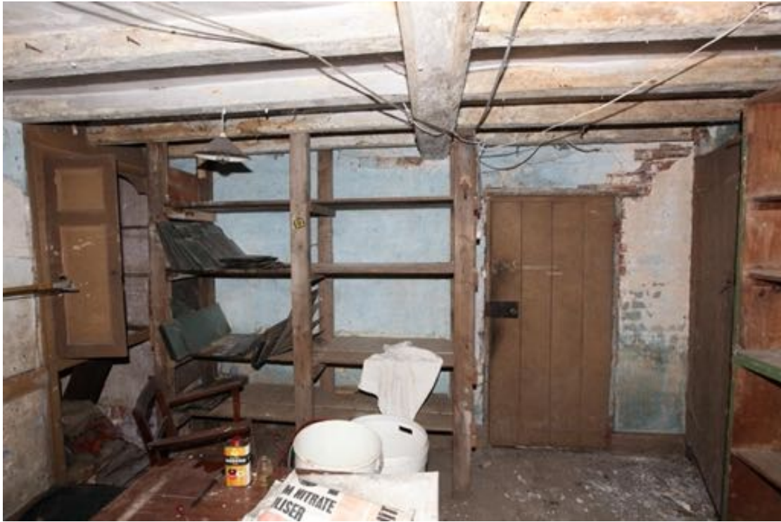
Illus. 19. The rear (northern) interior of the sitting room at no. 24 (G1) showing its lack of windows, exposed original brick fabric and the door to the lean-to 'garden room'.
