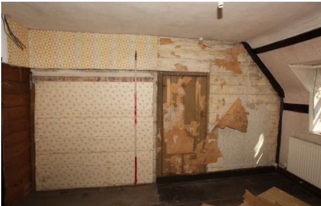
Illus. 46. The probably original first-floor partition between the western bedroom in no. 23 in the foreground and its counterpart to the east (F3). The horizontal deal boards are plain and the partition retains an original plank-and-batten door that was nailed shut and hidden behind wallpaper when the new staircase and extension were built. The door retains its probably original brown paint, matching that of no. 24.
