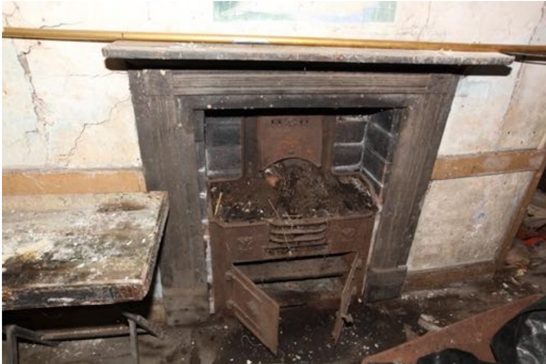
Illus. 15. A detail of the fireplace in illustration 14 showing its mid-19 th century reeded wooden fire surround with a slightly later hob grate and oven. The register plate is cast with the name of the manufacturer 'Cocksedge & Co. Ipswich', founded in 1879.
