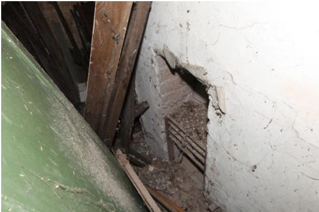
Illus. 34. A detail of the wrought iron basket grate in the western gable of the first-floor bedroom at no. 24 (F1).
