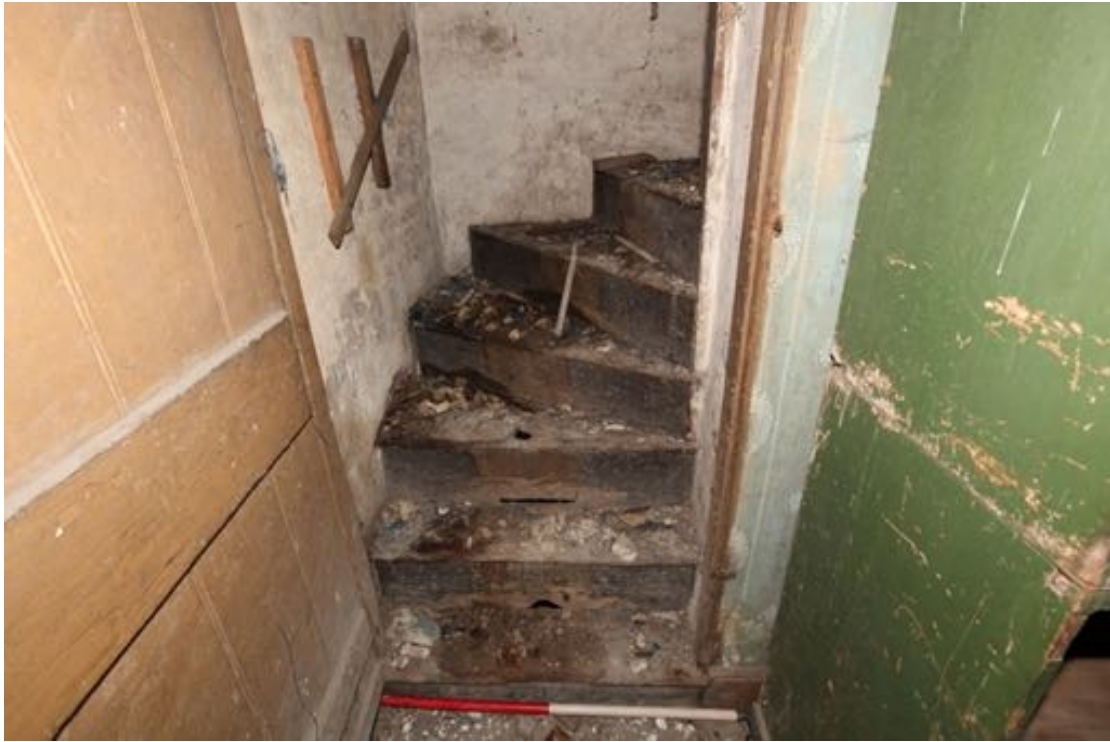
Illus. 23. The narrow original staircase of deal boards in the north-eastern corner of no. 24, as seen from the west (G1).
