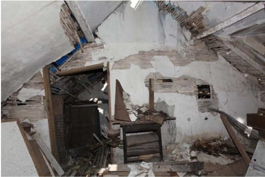
Illus. 35. The lath-and-plaster partition to the east of the first-floor bedroom in no. 24 showing the doorway to the stair landing on the left (F1).
