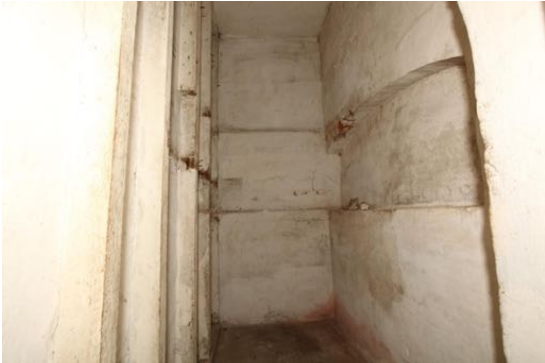
Illus. 45. The interior from the north of the cupboard that now occupies the position of the original bread oven with inserted narrow-sectioned studs adjoining the sitting room of no. 23 on the left. Any evidence of the oven is hidden by plaster. The arched shelf in the brickwork to the right adjoins the rear corner stair of no. 24.
