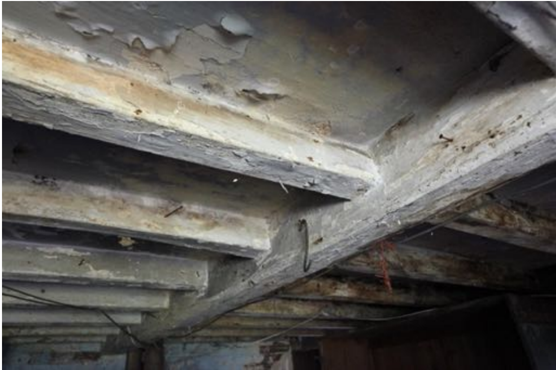
Illus. 17. A detail from the south-west of the original ground-floor ceiling joists of no. 24, showing the small chamfered edges that demonstrate they were intended to be visible as they remain (G1). The lath-and-plaster nailed to the undersides of the floorboards is also original. These narrow-sectioned joists of 4 ins by 3.5 are typical of the early- to mid-19 th century, but would have been rendered in houses of higher status.
