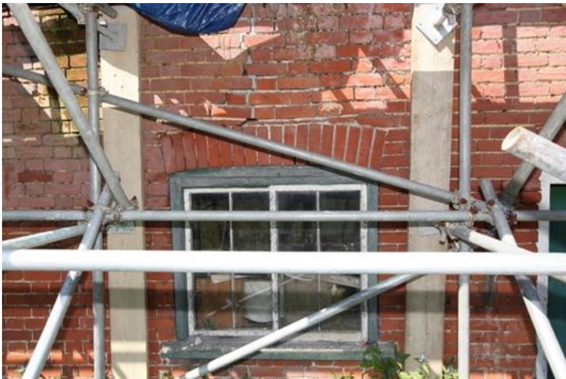
Illus. 4. A detail of the window to the left of the entrance door in illustration 2 showing its segmental arch and typically mid- to late 19 th century horizontal sash window. The brickwork is defined by closers (quarter-bricks) behind the scaffolding planks.
