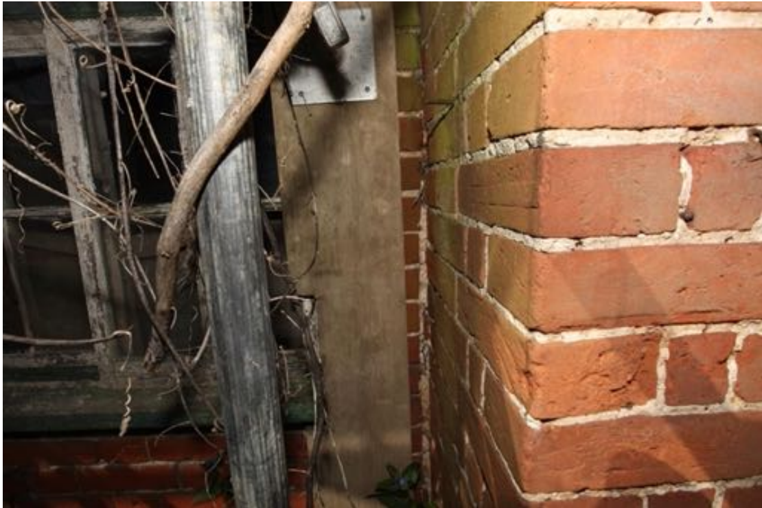
Illus. 5. A detail of the junction between nos. 24 on the left and 23 to the right, showing the mortar-filled vertical joint between their respective brick walls which demonstrates they were not built together. The 19 th century horizontal sash window of no. 24 is visible to the left.
