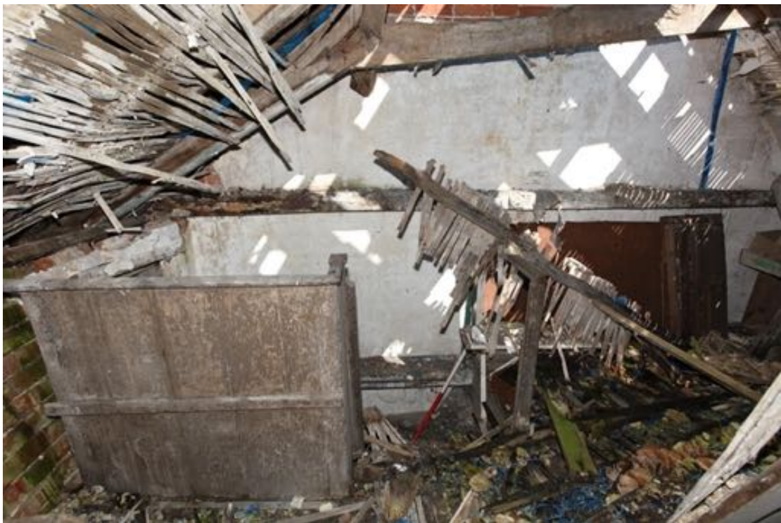
Illus. 30. The stair landing of no. 24 from the west showing the boarded partition against the corner stair on the left and the tie-beam abutting the rendered eastern gable in the rear (F2). The structure of no. 23 effectively borrows the brickwork of no. 24 and possesses no eastern gable of its own.
