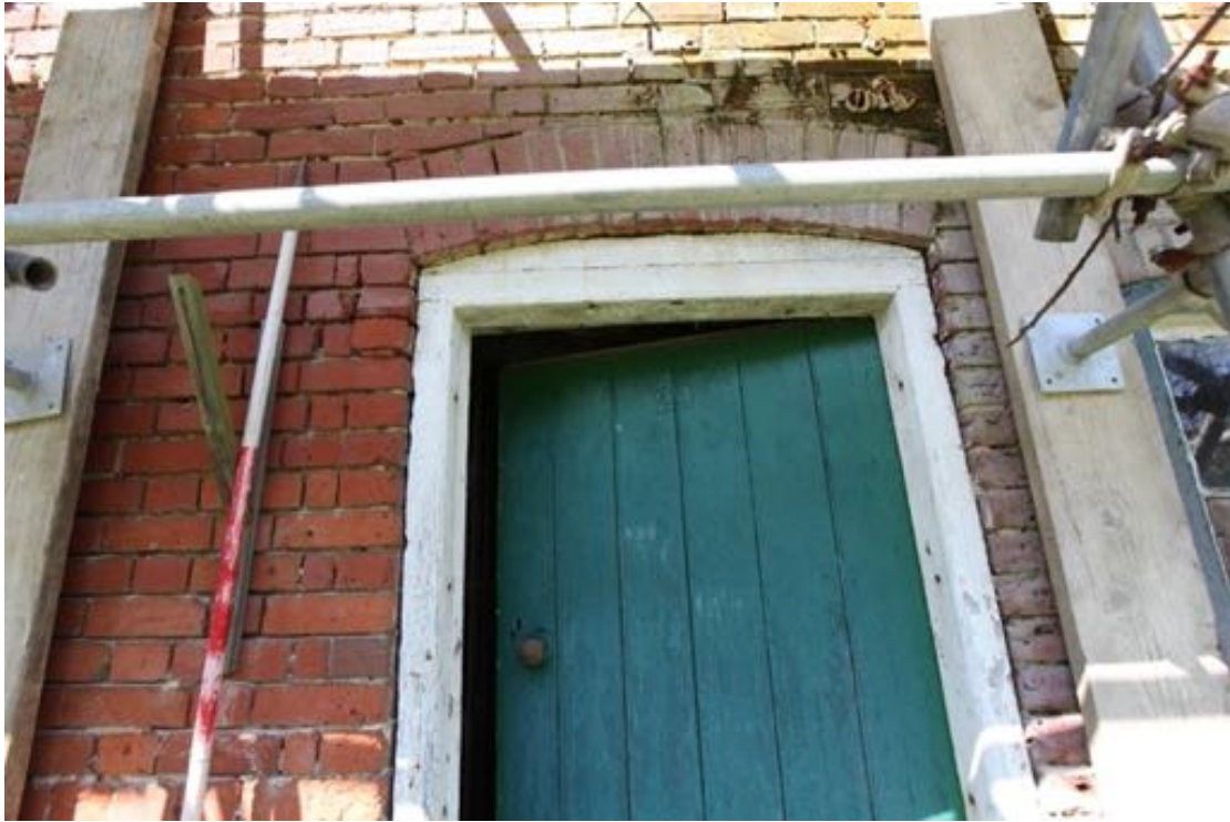
Illus. 3. A detail of what appears to be the original 19 th century plank-and-batten entrance door in the southern facade of no. 24, lacking a letter box but with the house number applied in cast numerals. The segmental brick arch contrasts with the horizontal tops of those at no. 23 and Lodge Cottage (indicating two separate phases of construction).
