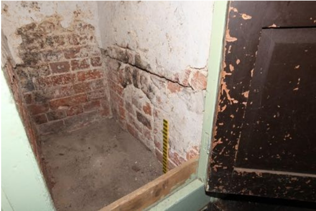
Illus. 41. A detail of the right-hand pier of the original wider fireplace in illustration 40 showing the blocked arch of an ash hole under a bread oven (into which the hot ashes of the faggots would have been raked after heating the oven). The soldier course above formed the oven floor but its aperture is hidden by plaster above. The position of the oven is now occupied by the storage cupboard in illustration 45.
