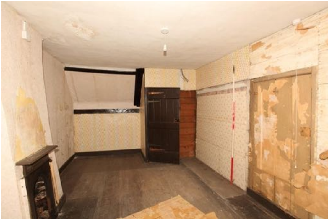
Illus. 47. The western bedroom of no. 23 seen from the south (F3), with the blocked door of the original internal boarded partition on the right and the late-19 th or early-20 th century cast iron coal grate of its western fireplace on the left. The roof-structure of staggered butt-purlins is visible to the left of the early-20 th century internal porch which opens onto the new stair and rear bedroom of the same period.
