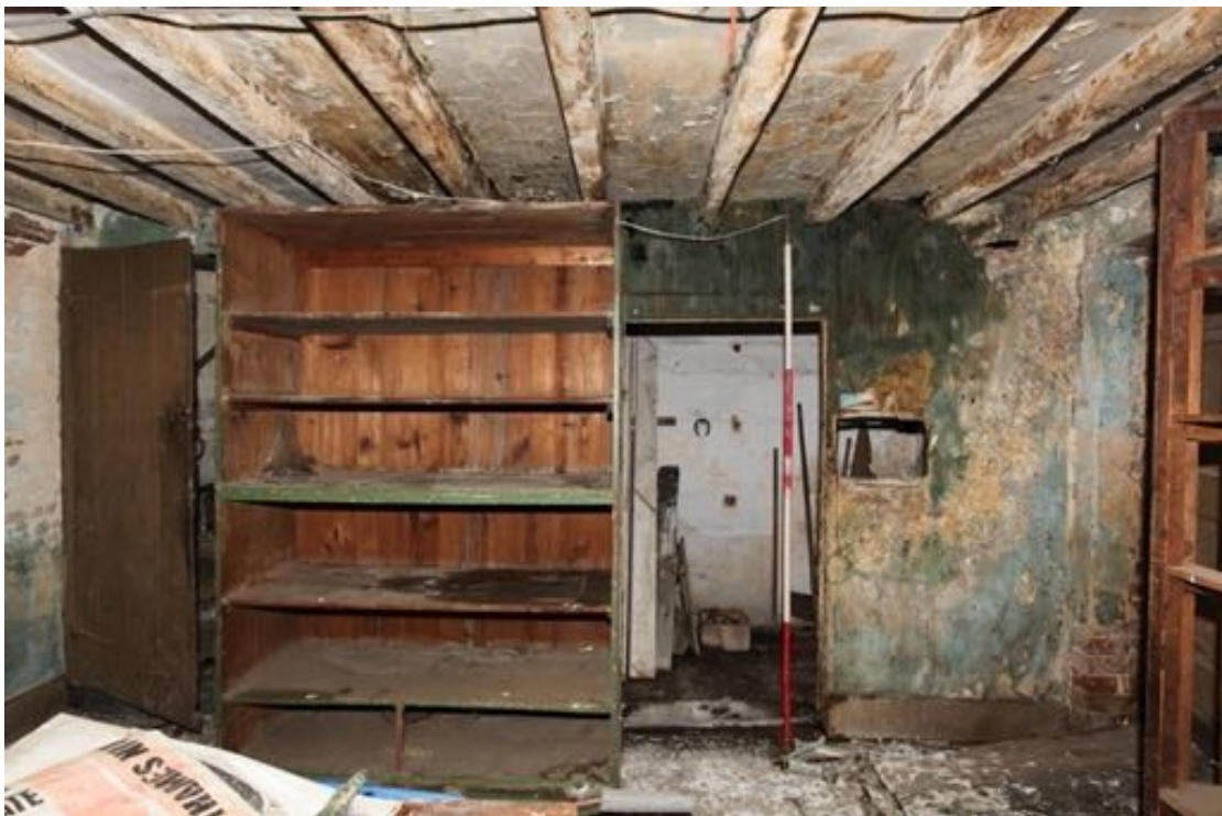
Illus. 18. The eastern wall of the sitting room at no 24 (G1) showing the stair door on the left and the entrance to the storage cupboard in front of the stair (G2). A set of storage shelves bearing old green paint divides the two.
