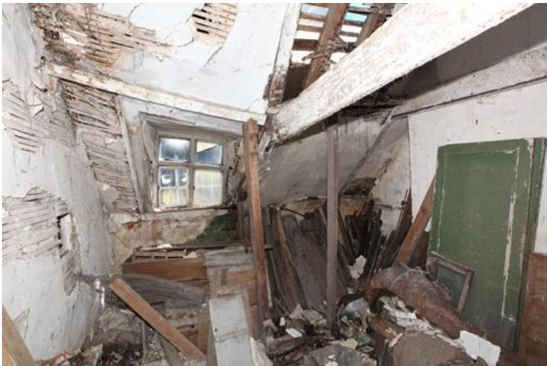
Illus. 32. The first-floor bedroom at no. 24 from the north (F1), showing its dormer window and the lath-and-plaster ceiling which extends to the apex of the roof. Nails in the underside of the roof collar indicate that an earlier lower ceiling matched that of the stair landing to the east.
