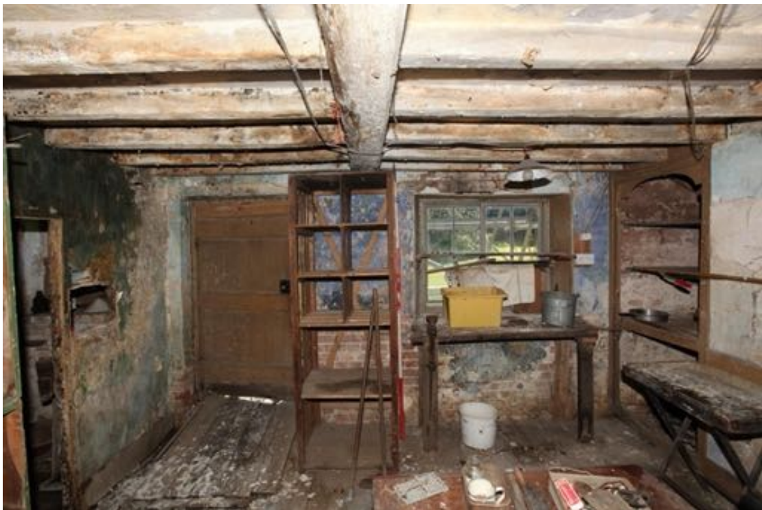
Illus. 16. The southern internal ground-floor wall of no. 24 showing the storage area in front of the stair (G2) and the entrance door on the left with the horizontal sash window and arched cupboard to the right (G1). The external walls consist entirely of 35 cm 19 th century brickwork visible here beneath the window and there is no trace of earlier fabric.
