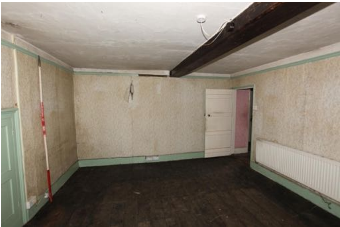
Illus. 42. The rear (northern) wall of the sitting room at no. 23 (G5) showing the chamfered pine binding joist of the original ceiling and the outline of a blocked door to its left. This doorway is likely to have opened into the lean-to that pre-dated the present kitchen extension and is also indicated by an insert in the skirting board.
