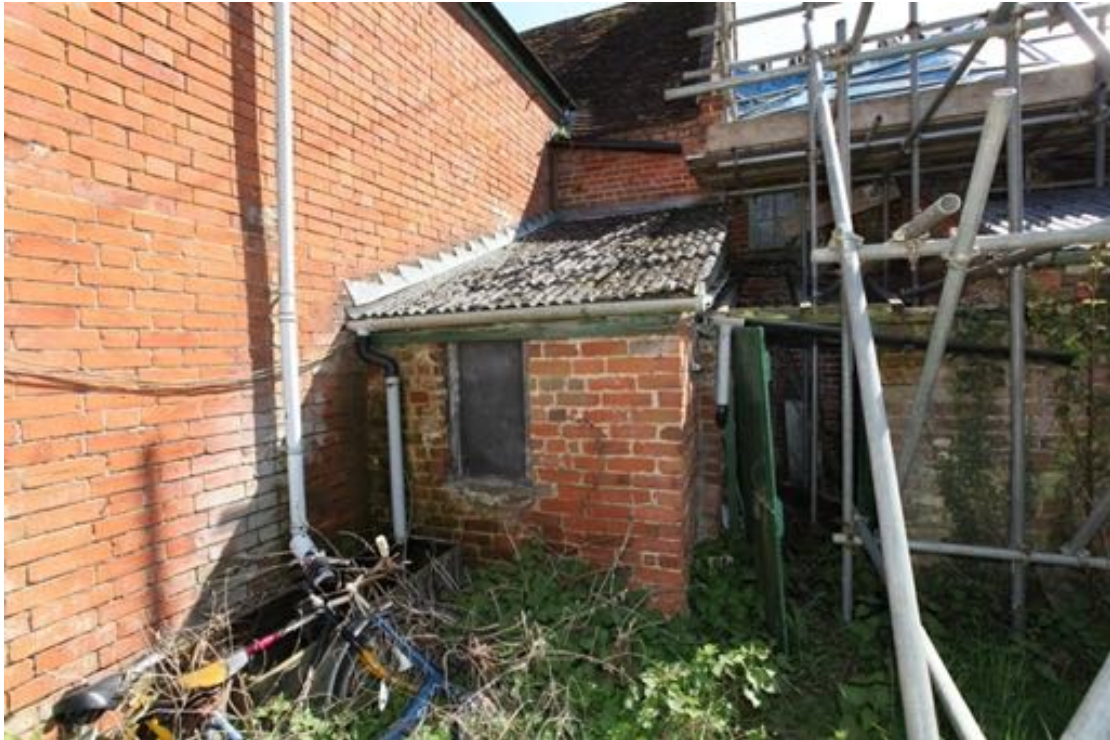
Illus. 9. The lean-to larder of no. 23 in the north-eastern angle of the southern range and its early-20 th century rear extension (G7). This appears to represent a fragment of the mid-19 th century lean-to that extended further to the left prior to the construction of the extension. It is adjoined on the right by a narrow gap, now enclosed by a door, with the lean-to of no. 24 to the extreme right.
