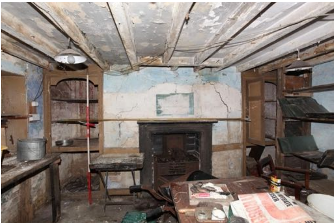
Illus. 14. The ground-floor fireplace in the western gable of no. 24 flanked by identical pairs of cupboards retaining their probably 19 th century paint scheme of light and dark brown (G1). The original cupboard doors survive in part to the right and hinges remain on the left.
