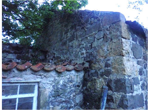
Crevices in the masonry
