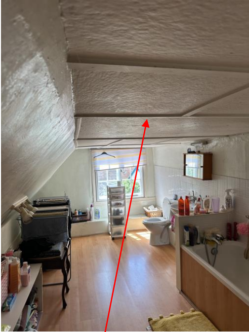
2 nd Floor bathroom. The ceiling we are proposing to raise in height
