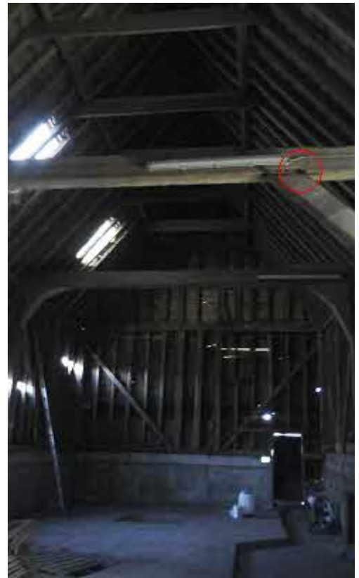
Tn 3. Traditional barn exterior, and interior structure; bat roost circled in red.
