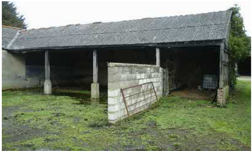
Tn 4. Dilapidated livestock buildings and yard area.
