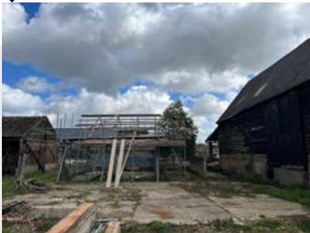
Extension off the rear of the barn (Collapsed)
