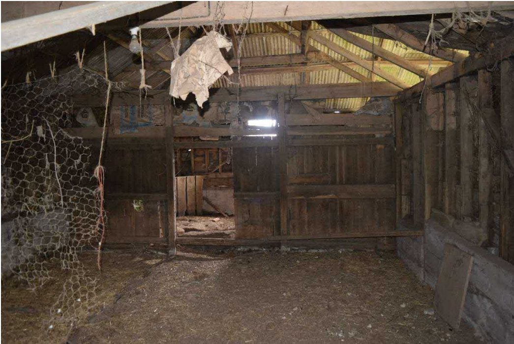
Figure 28: Shed attached to the North-East end of the C19/C20 open-fronted shelter shed.
