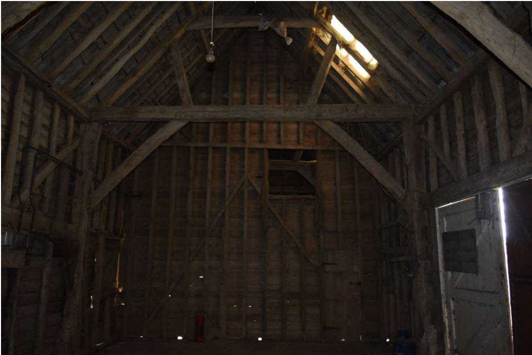
Figure 23: Interior view of the stable barn towards the South-West, showing the inserted partition wall.
