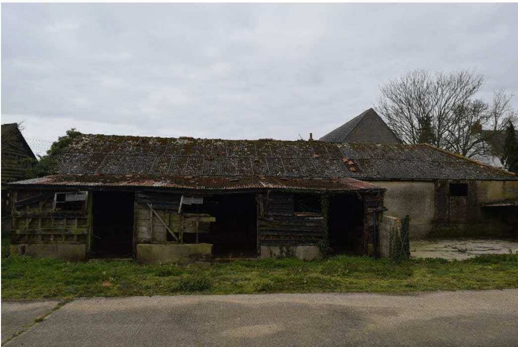
Figure 29: 3-Bay animal shelter attached to the rear of the North-East end shelter shed.
