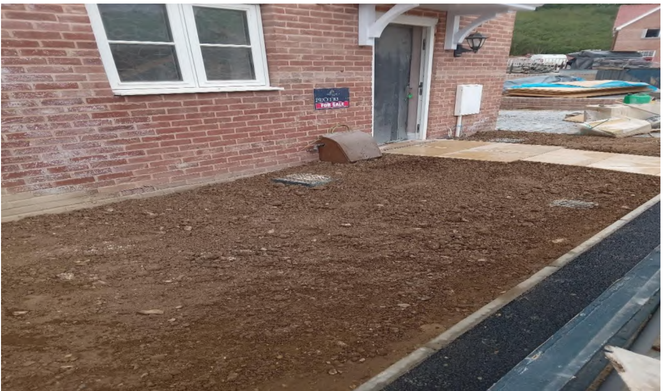
Client Supplied Photographs 13-15 , taken on the 31 st May 2023 showing topsoil placement within the front gardens of plots 80-83.
