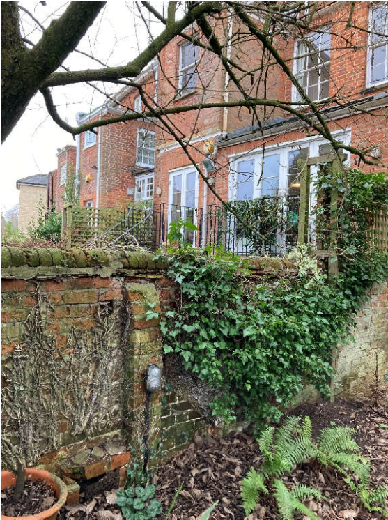
Neighbouring extensions, crumbling garden wall
