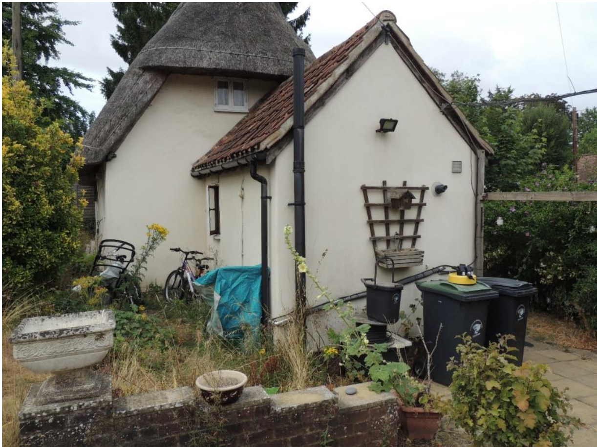
Photo 1: Looking southwards at the site. The proposal is to demolish part of the existing extension and erect a larger one that would extend to the east and north
