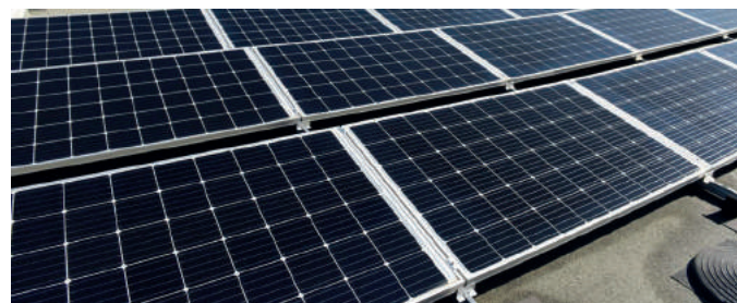
Photovoltaic panels on main flat roof
