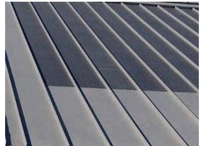
Thin film PV panels (on inner south-facing roof slope)
