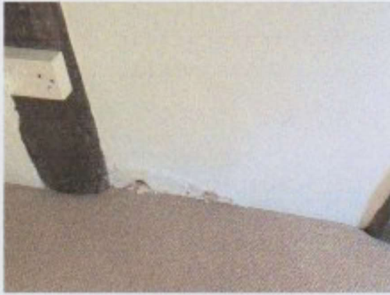
Photo 3: close-up of panel deterioration.
