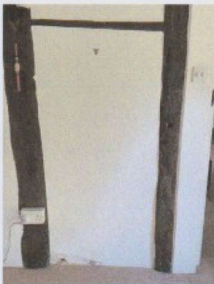
Photo 2: panel showing deterioration in lower part.
