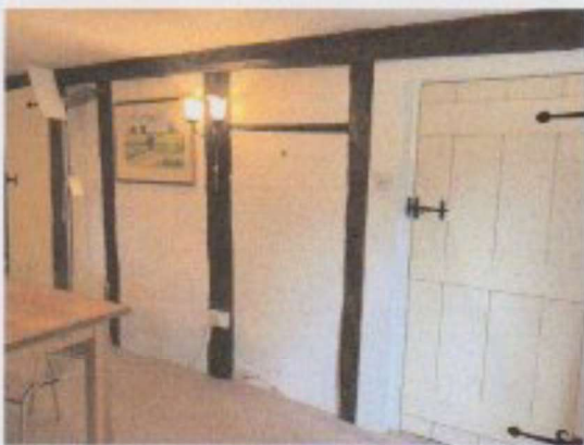
Photo 1: plasterboard panel to be removed (to right of wall light, below horizontal bar).
