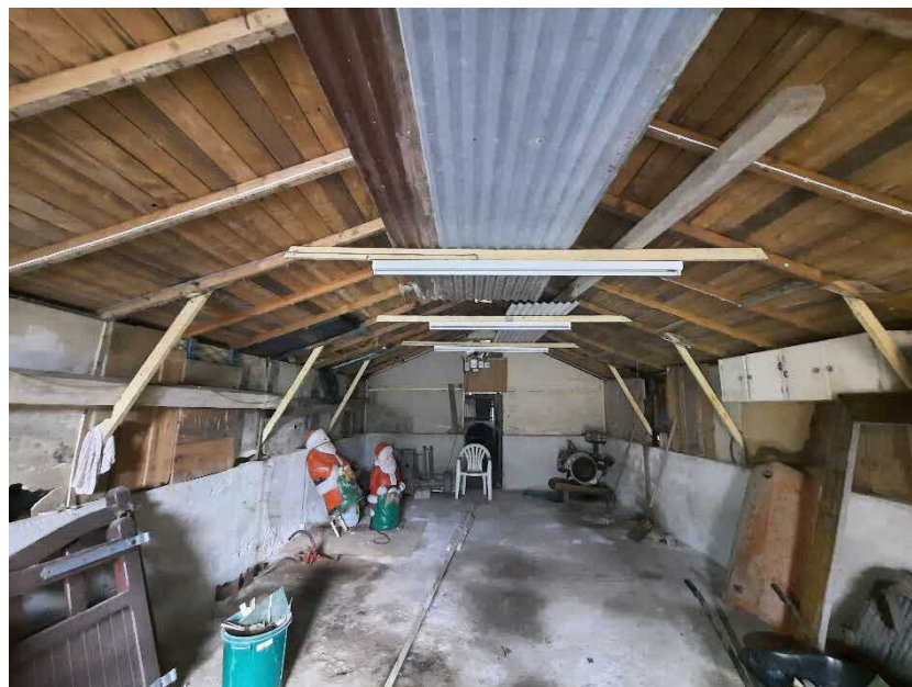
Figure 4: Interior view (towards east) of the timber garage at Vigus Stores, showing the unlined timber sheet roof and stored items.
