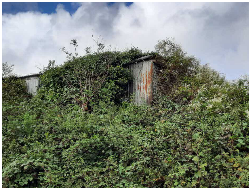
Figure 8: View (towards north) of the vegetation encroaching much of the southeast corner of the workshop at Vigus Stores.
