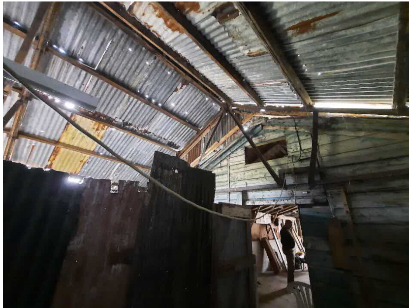
Figure 5: Interior view (towards west) of the corrugated extension to the east of the timber garage at Vigus Stores, showing the unlined corrugated metal sheet roof and timber partitions present.
