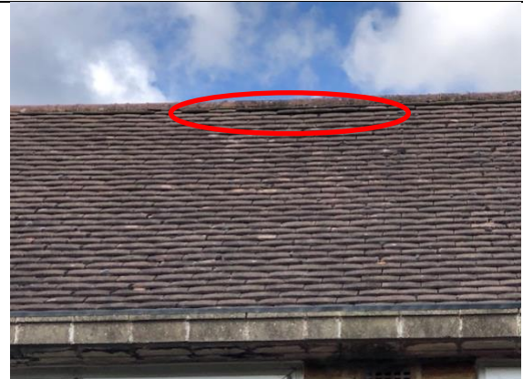
Photograph 4: There were minor gaps under a few of the tiles just below the ridge line – no proposed work in this area and not considered large enough to support roosting bats.
