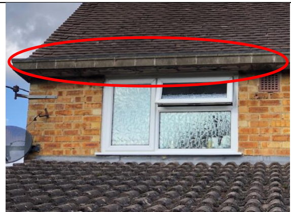
Photograph 6: The soffits on the rear elevation were of concrete breeze block construction and presented no gaps or potential roost features (PRFs) for bats.
