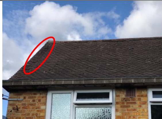
Photograph 3: The rear roof of the property. Red circle illustrates some very minor gaps under a few of the roof tiles along the edge of the roof. Not considered large enough to support roosting bats.
