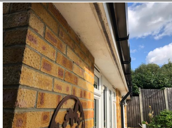
Photograph 7: The wooden soffits on the single-storey rear extension presented no gaps or PRFs for bats.
