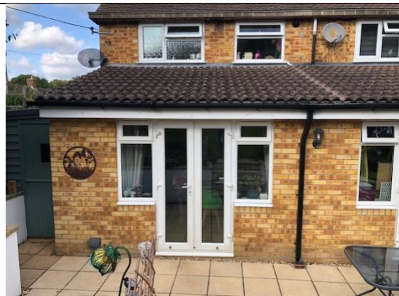
Photograph 5: Part of the single storey rear extension. There were no gaps under any tiles on this part of the roof.
