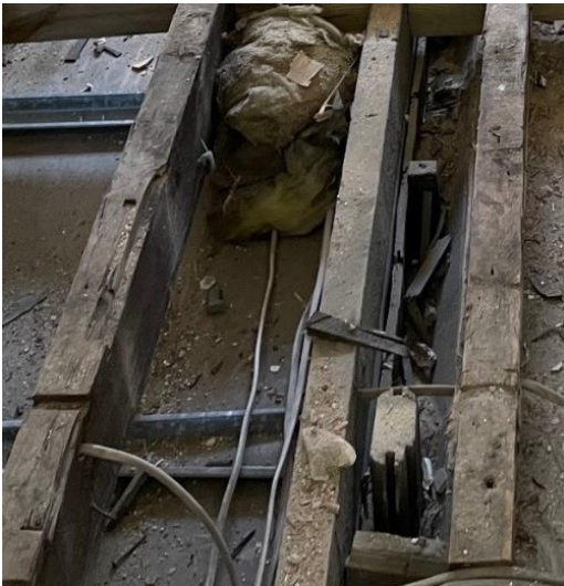
Image 04: Existing floor levelling attempts illustrating firrings and a combination of timber laths to the existing joists showing the plasterboard ceiling on resilient bars to the ground floor commercial unit.
