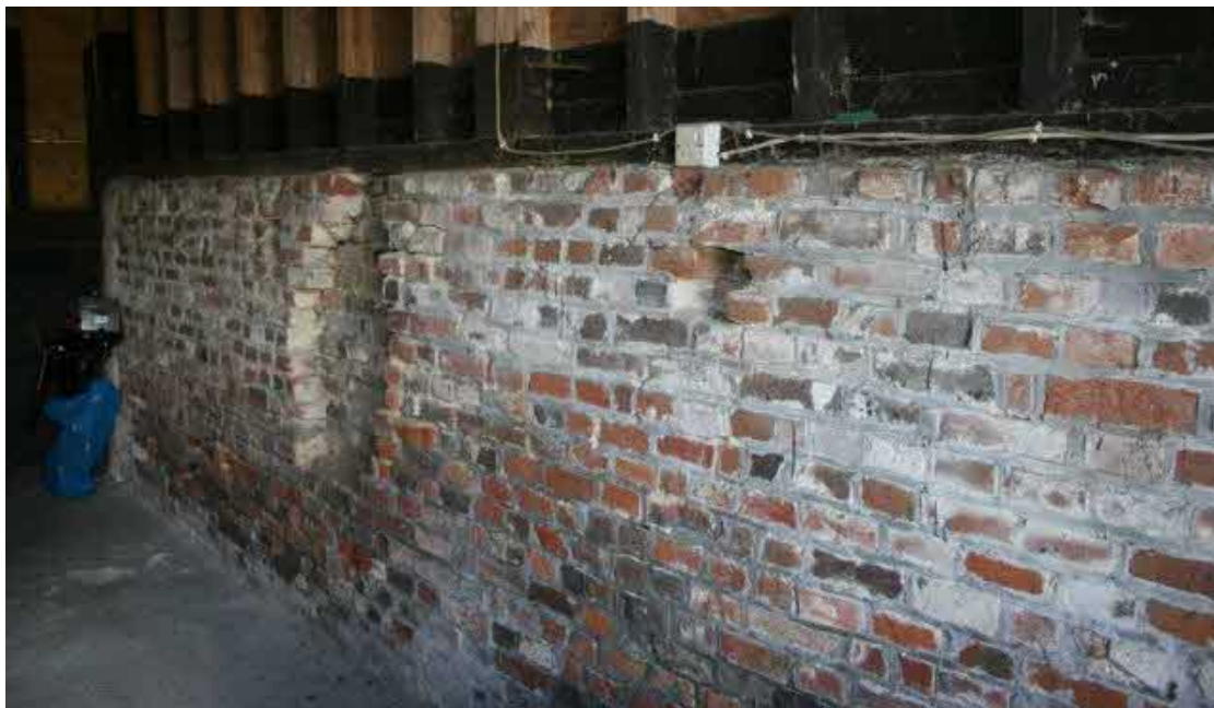
The partition is made from reused C19th bricks set in grey cement.
