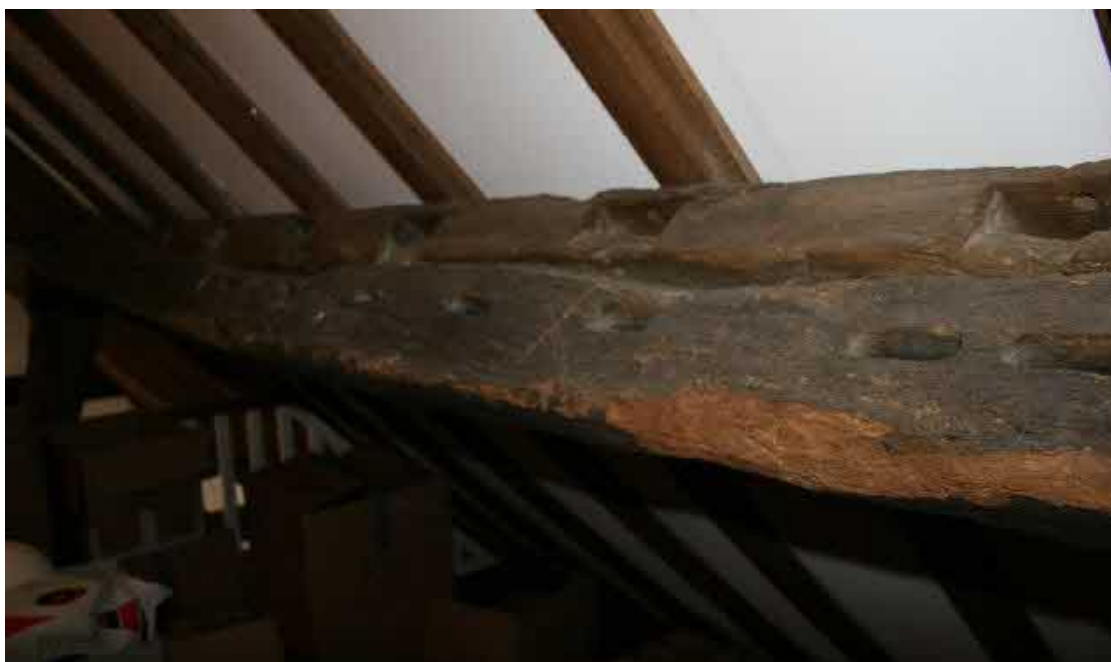
Detail of doubled up purlins made from top-plates on the north side of the mezzanine.
