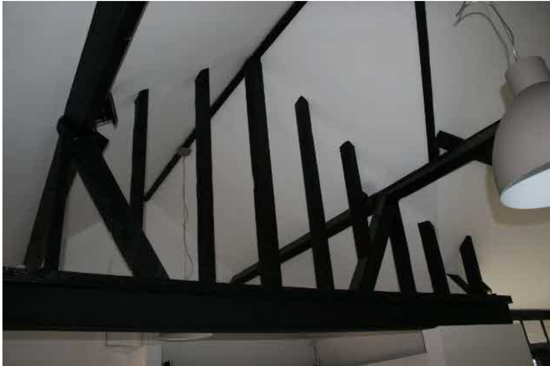
Detail of the southern truss. Only the principal timbers are C19th. Looking SW.
