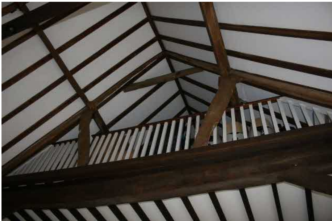
Looking up at the mezzanine floor. The queen posts appear upside down.
