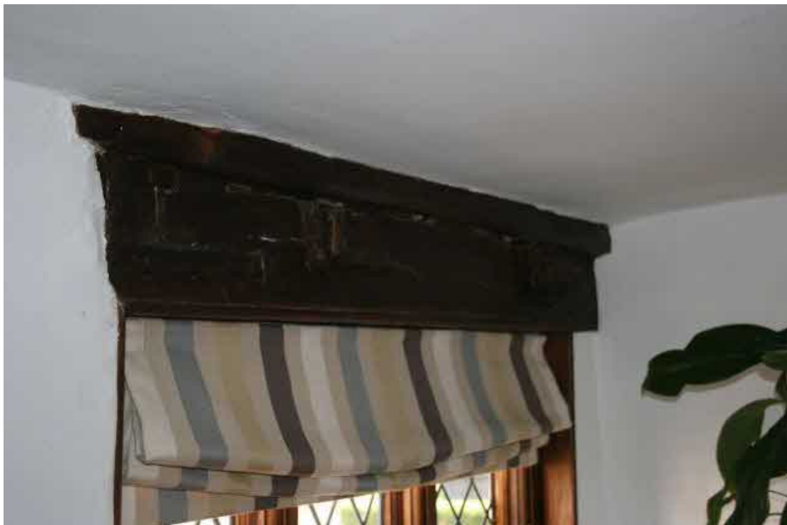
Two large metal staples are fixed to the frame over the window.
