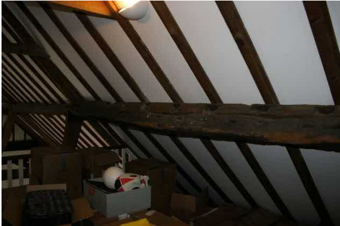
Doubled up purlins made from top-plates on the north side of the mezzanine.
