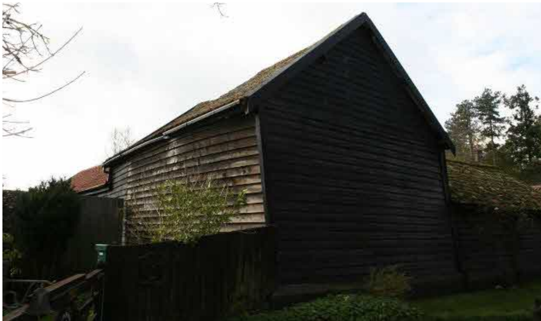
The south and east elevations of the Workshop. The building borders the neighbour's garden.
