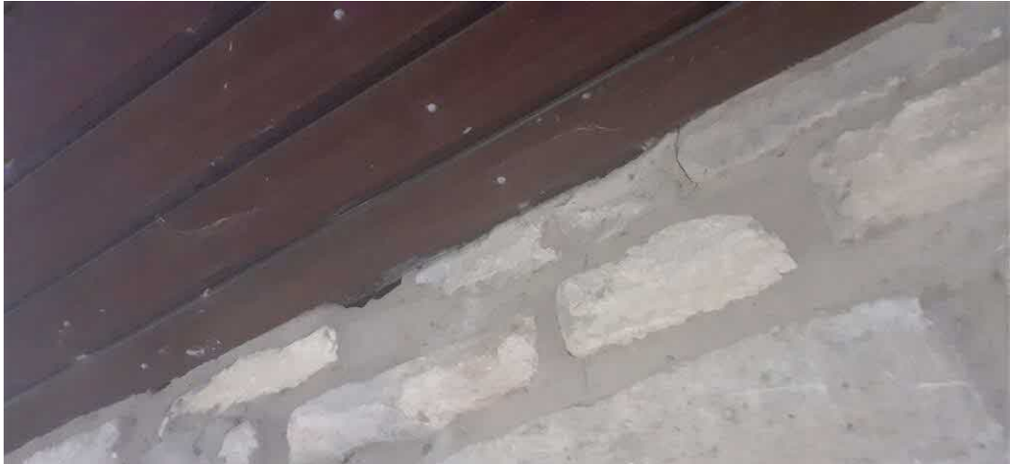
Plates 6: View of a gap on the western side of the building
