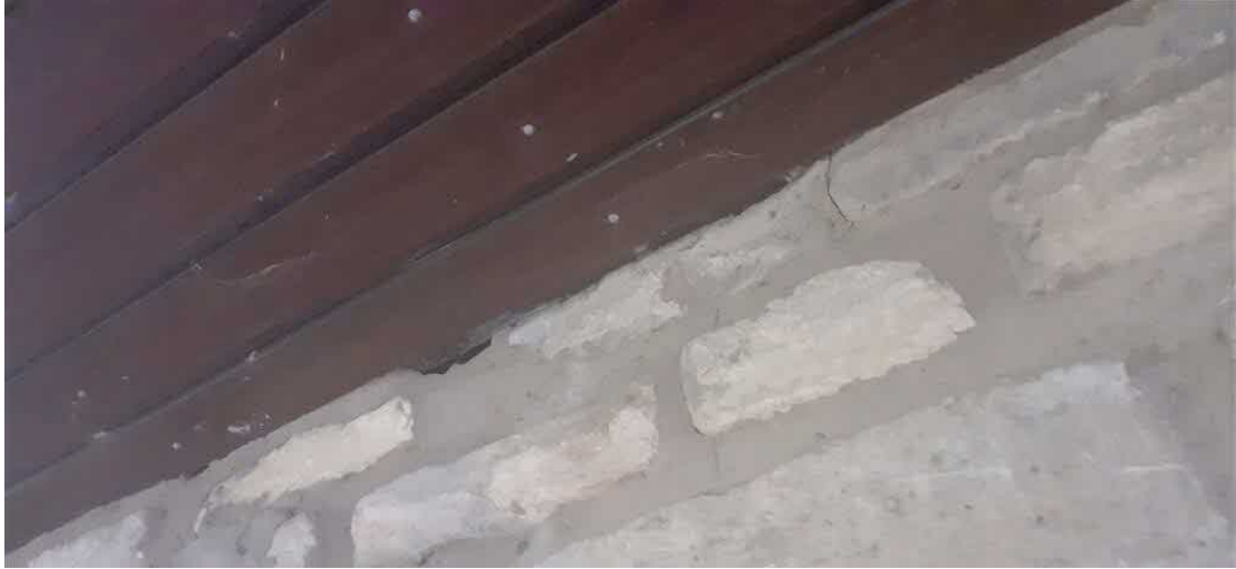
Plates 6: View of a gap on the western side of the building
