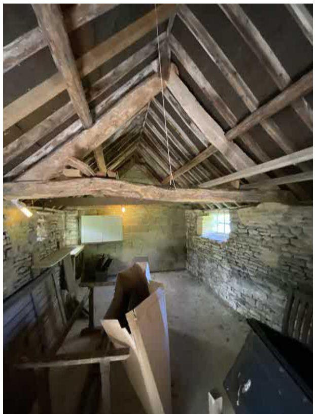
outbuilding - existing stonework repaired and repointed, blockwork party wall dry-lined in new shower room at end - modern concrete slab floor rained or replaced tbc
