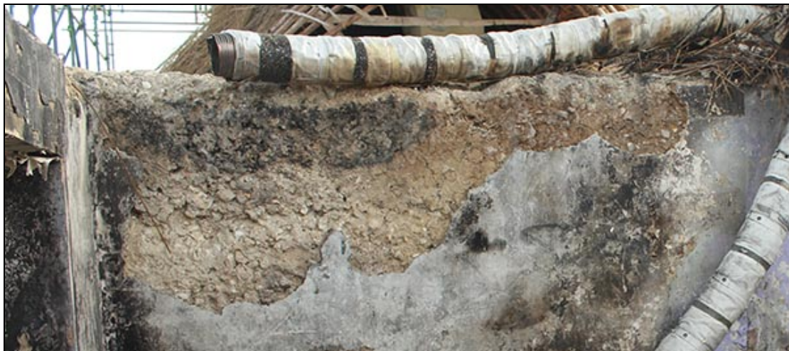
Figure 12 Exposed section of cob walling in first floor rear room of No.1, looking east
