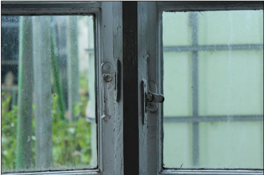
Figure 28 Two of the three surviving Phase 3 window catches, here in the rear room of No.2
