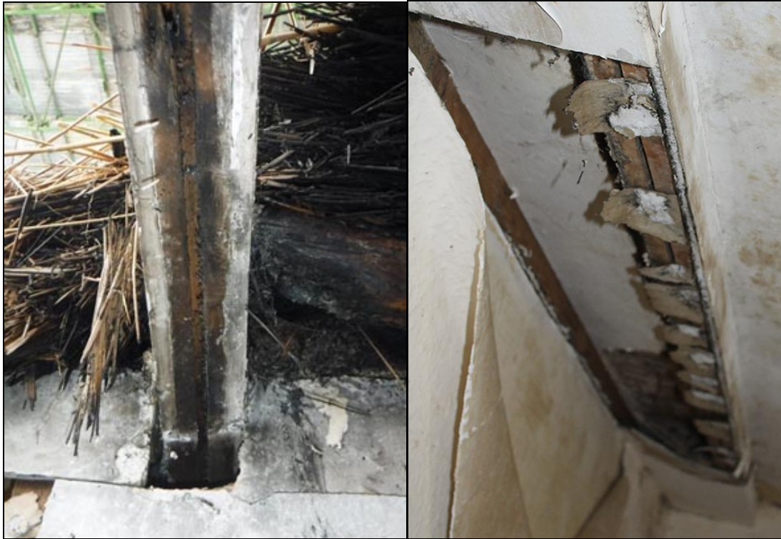
Figure 20 The grooved timbers in the first floor ceilings that once accommodated thin boarded partitions. To the left is the east-west running one in No.2 (looking east), and to the right is the north-south running example in No.3 (looking north)
