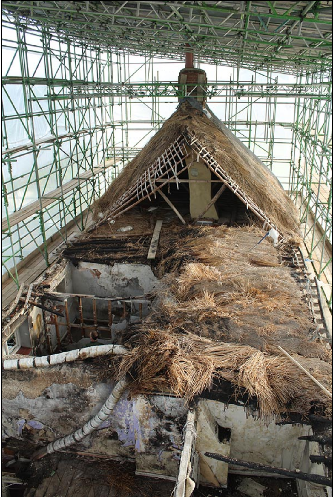
Figure 10 The remains of the roof of the Barracks, looking east. The fire damage progressively gets worse from No.1, in the foreground, through No.2, which still retains the frame of its studwork in its upper rear rooms, to No.3, where the internal rooms are largely intact, to No.4, where there is little visible damage.
