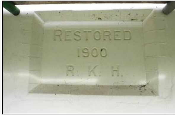
Figure 23 The restoration stone centrally set into the south face of the cottages
