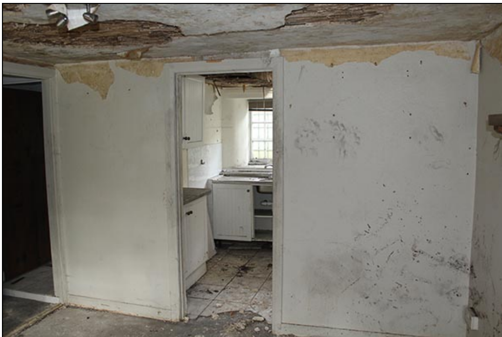
Figure 34 The Phase 4 ground floor internal partitions dividing the rear space into bathroom (to the left), kitchen (centre) and pantry/cupboards, here in No.1.
