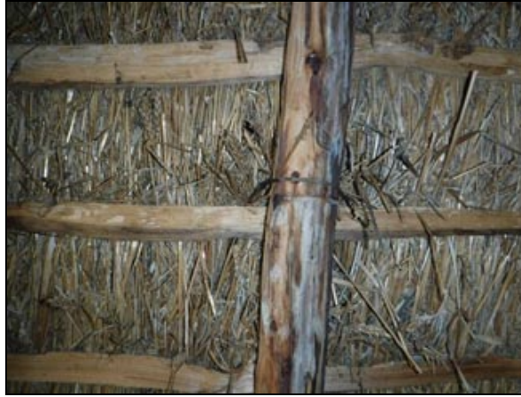
Figure 18 Detail of the inside of the roof, showing the cleft oak laths and tarred twine, used to fix the base coat of the straw
