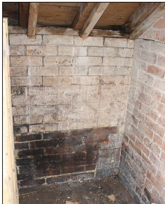
Figure 25 The infilled brickwork in the rear wall of the northern of the two eastern privies, indicating the location of a hole that once may have been linked to a pig-sty behind
