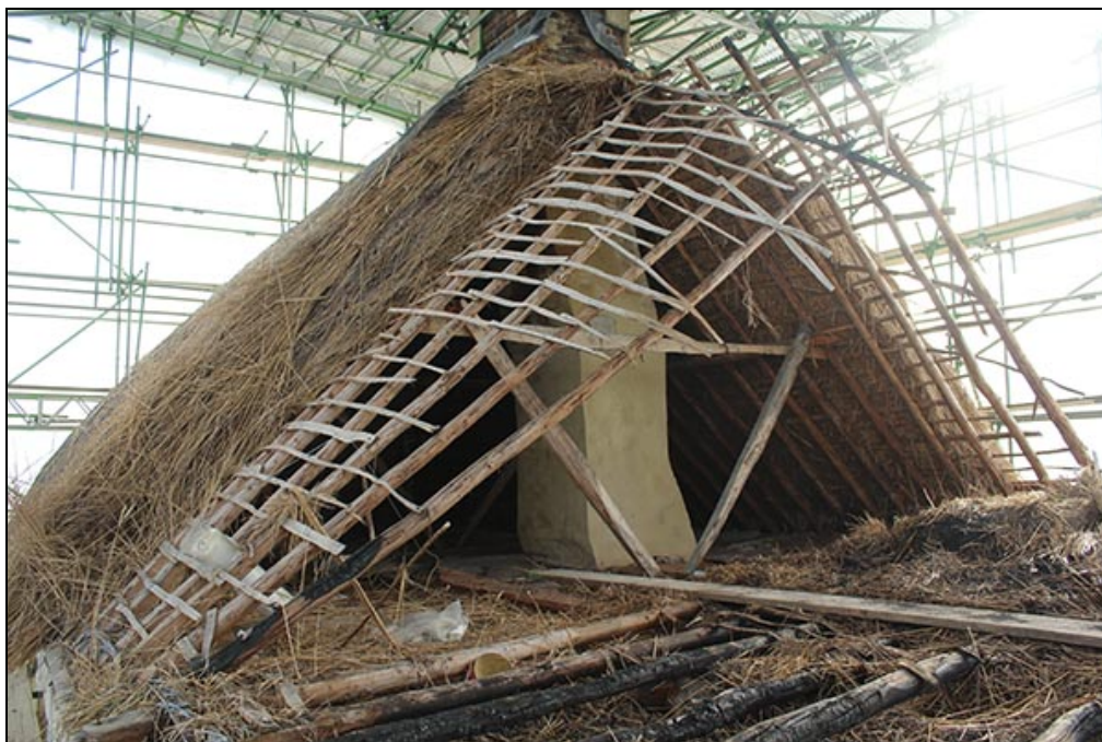
Figure 17 The surviving section of roof over No.4, showing its construction, looking east
