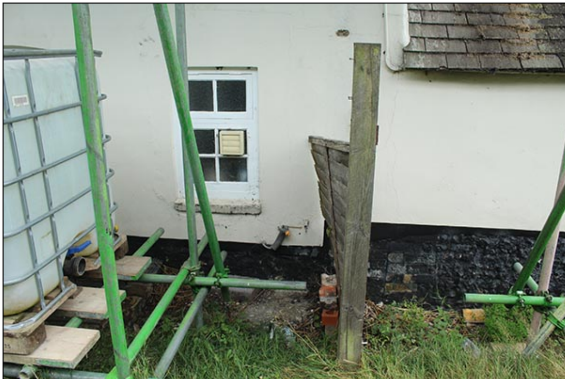
Figure 14 The dwarf wall supporting the cob of the cottages (to the left of the wooden fence) and the higher level one supporting the walls of the western outshot (to the right)
