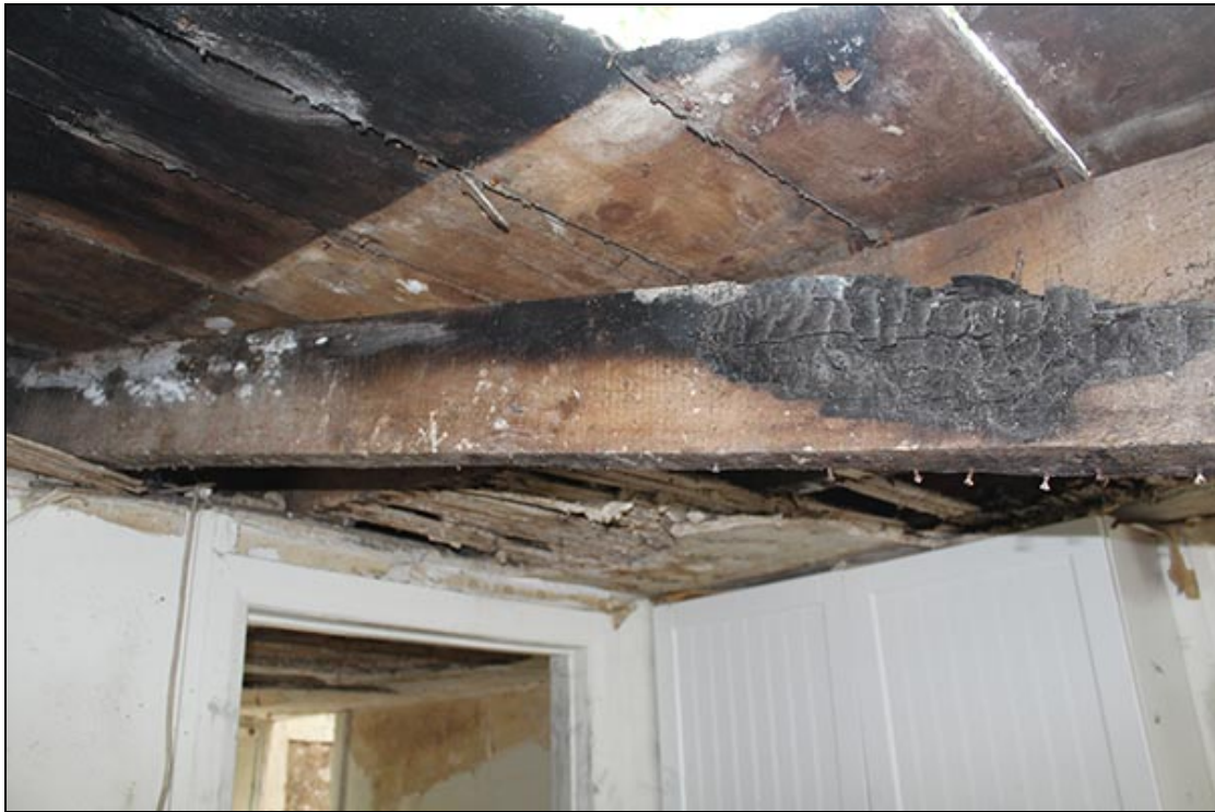
Figure 19 The northern first floor poplar joists, here still partly supported on the dividing wall between the two ground floor rooms in No.1, with the elm floor boards above, and a remnant of the lath and plaster in the corner, looking south-west
