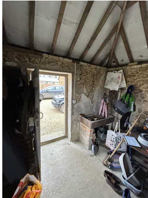
Photo North End of Outbuilding indicating brand new roof timbers and breathable membrane with Sink and hand pump in the corner
