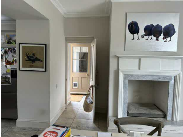
Photo of fireplace and wall to be removed Central wall nib to be removed (left of picture)
