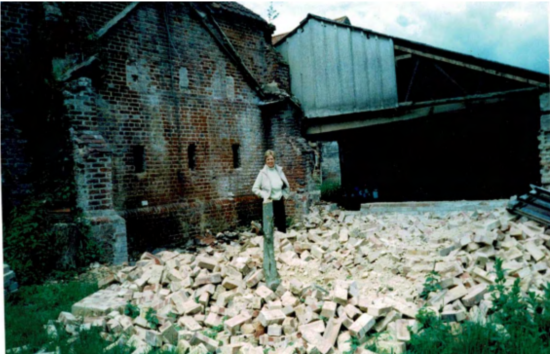
Plate 7 - Photograph taken during the conversion of the north-east corner of the main barn. The attached garage is within the right hand structure that was further reduced in size from what is photographed.
