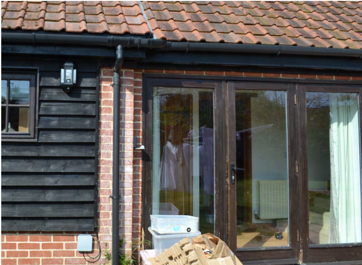
Plate 11 - Example of fenestration requiring replacement (D1001)
