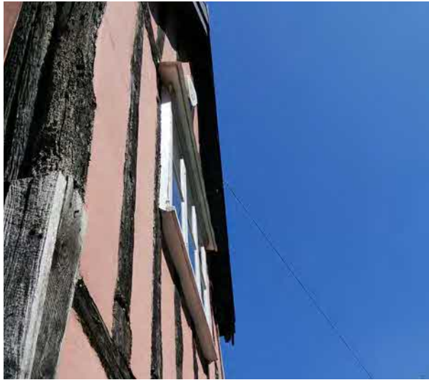
First floor western crossing 19th Century window, showing 60mm protrusion beyond timber frame
