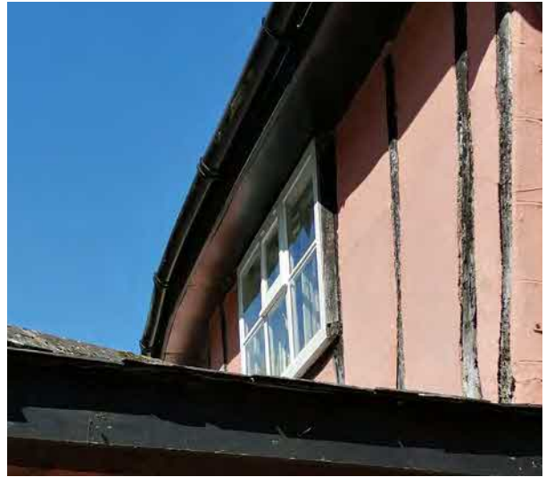
19th Century window above butcher's shop roof, showing 50mm protrusion beyond timber frame
