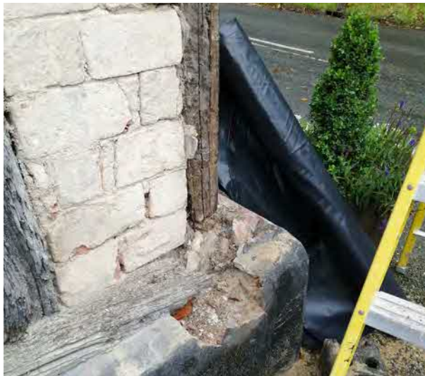
Southwestern corner of house, showing required repair/strengthening of corner post and sole plate
