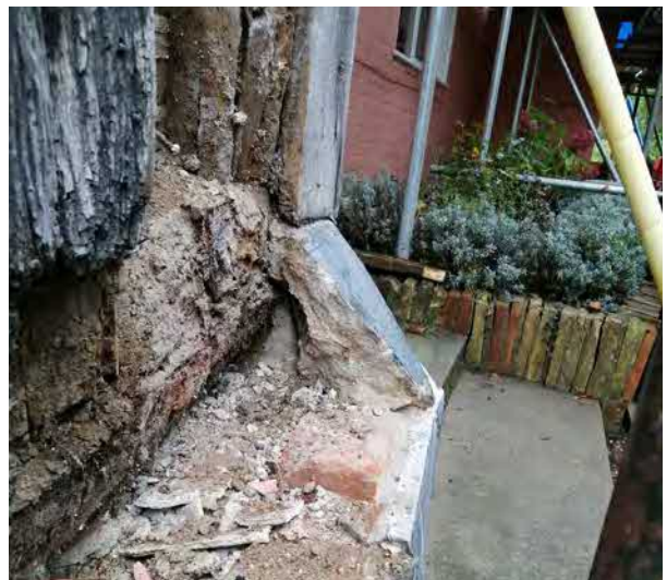
Decayed sole plate at south side of western crossing to be replaced
