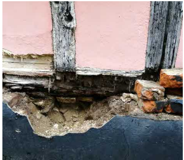
Decayed sole plate at south side of western crossing to be replaced
