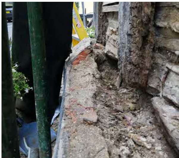
Concrete and brick plinth at south side of western crossing currently traps water against sole plate
