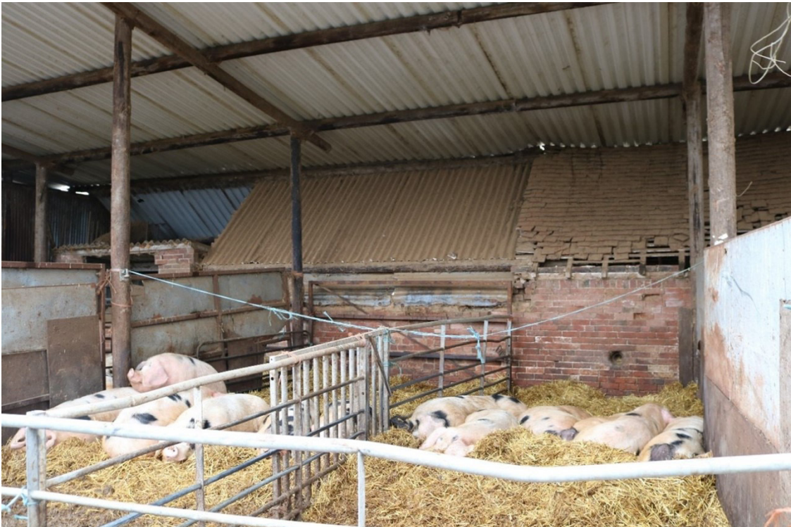
Image EDP A2.8: View westward toward L-shape range at Southview Farm, showing its partial incorporation into a modern farm building.
