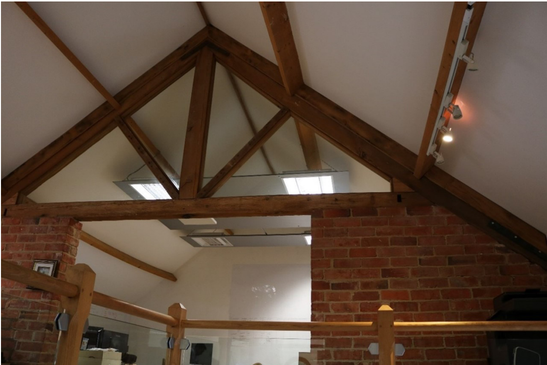
Image EDP A2.6: Internal view of Camp Farm barn modern roof structure.
