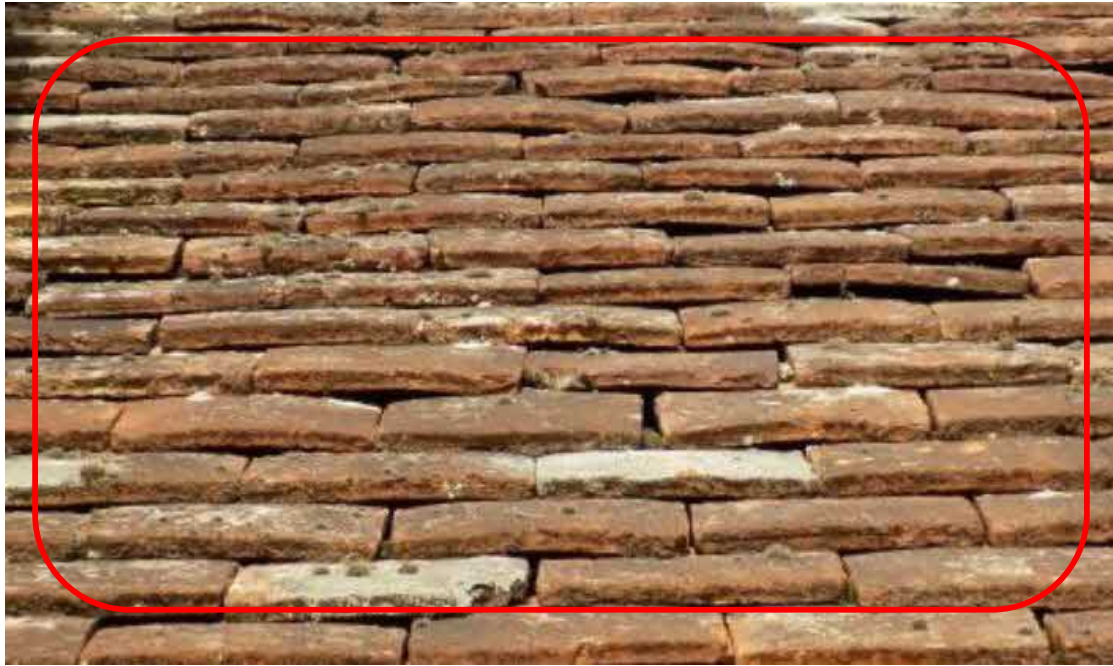
Image 7 – East facing connecting roof coverings between the building and main dwelling which has demonstrated gaps of value to bats
