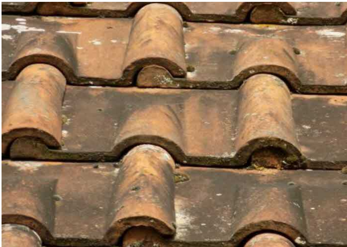
Image 2 – Close view of the West facing roof coverings which have demonstrated a fair level of condition
