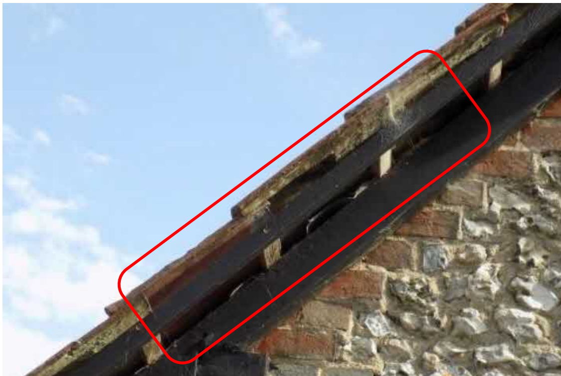
Image 4 – North facing gable offering gaps to the eaves areas which look to offer likely access opportunities for bats
