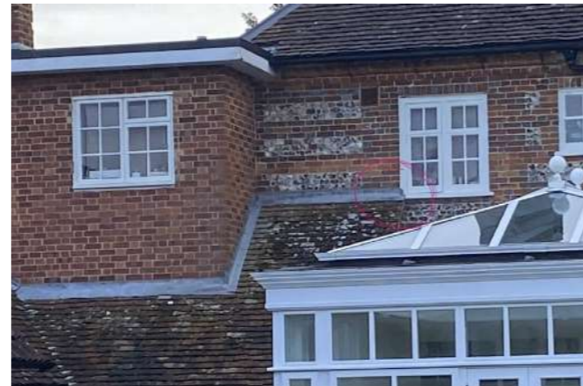
Remnants of catslide roof, awkwardly abutting original window at first floor level.
