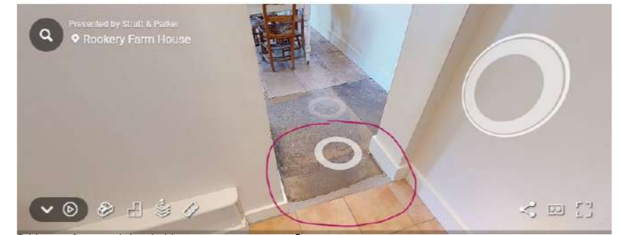
Evidence of external threshold
