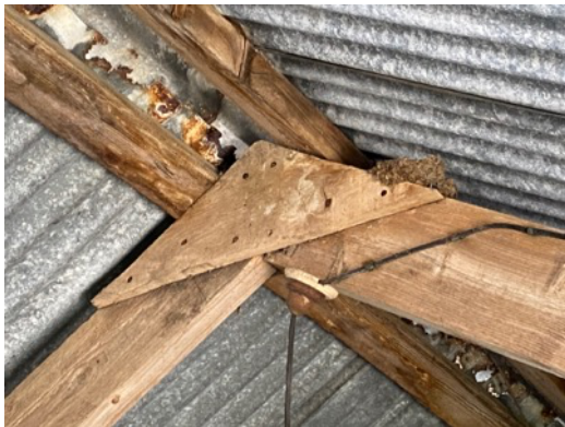
Photo 11: B3 – internal view of roof structure showing lack of underlining, and inactive bird nest.
