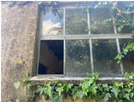
Photo 21: B5 - absent window pane at south-eastern gable end.
