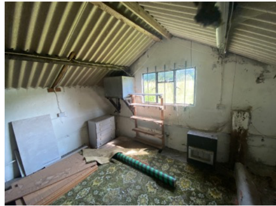
Photo 14: B4 – Internal view showing significant light spillage.
