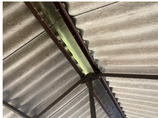
Photo 6: B1 – internal view of roof structure with light ingress from ridgeline vents.
