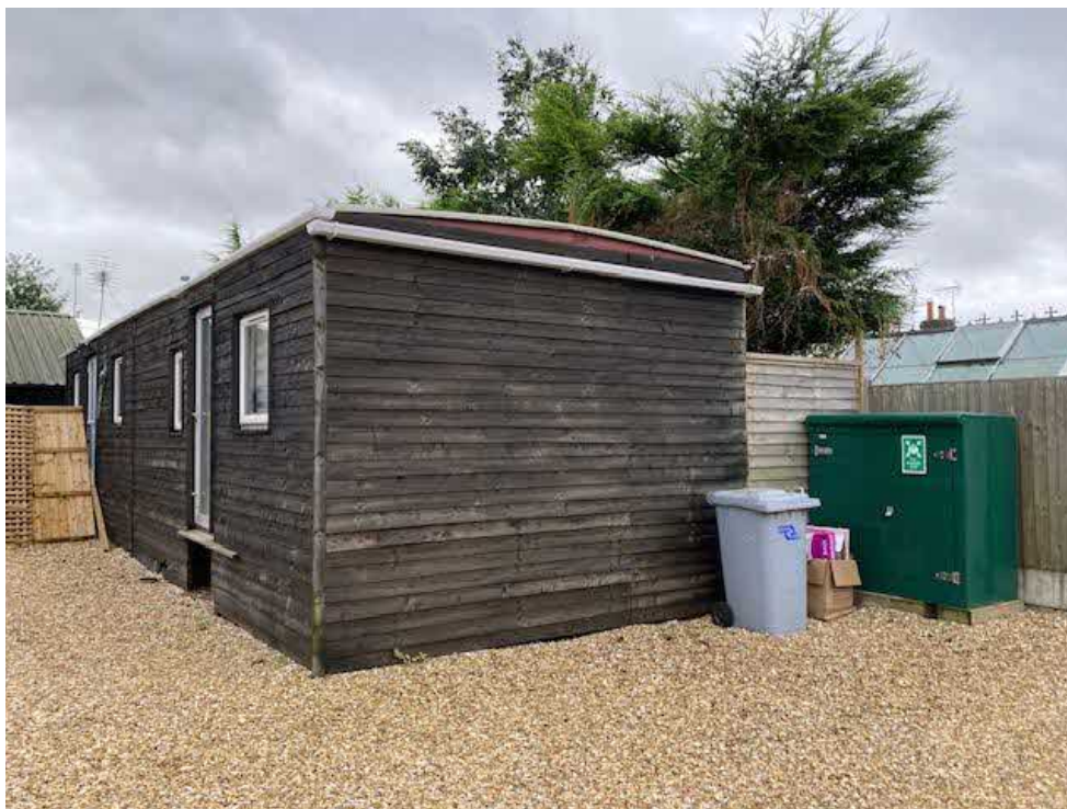
25. The north west end of the cabin amenity building and rear timber fence.
