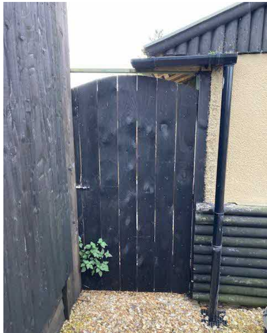
6. The timber boarded gate at the rear east corner of the amenity building.
