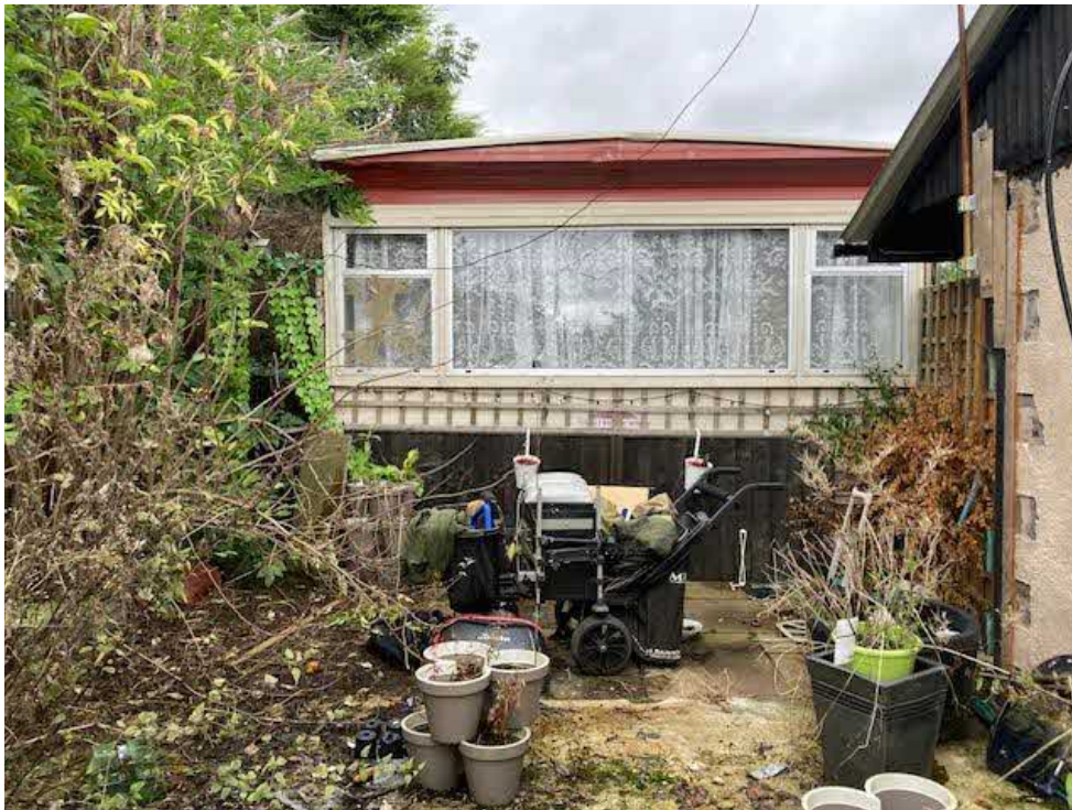
27. The large window in the south east end of the amenity cabin building.
