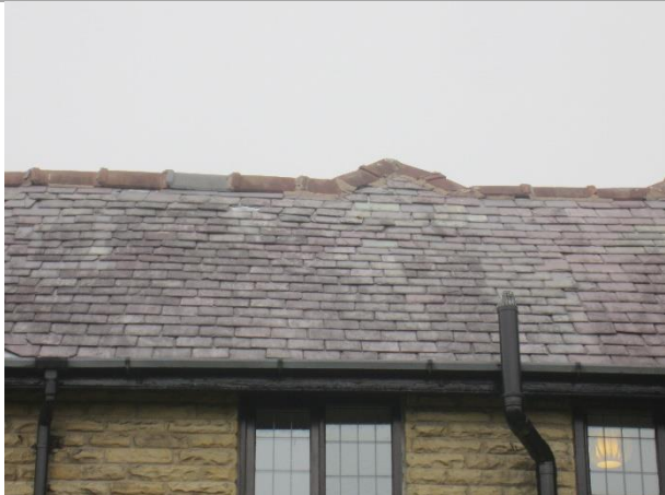
Photo 11: Slate covered roof at the farmhouse showing highest points of void
