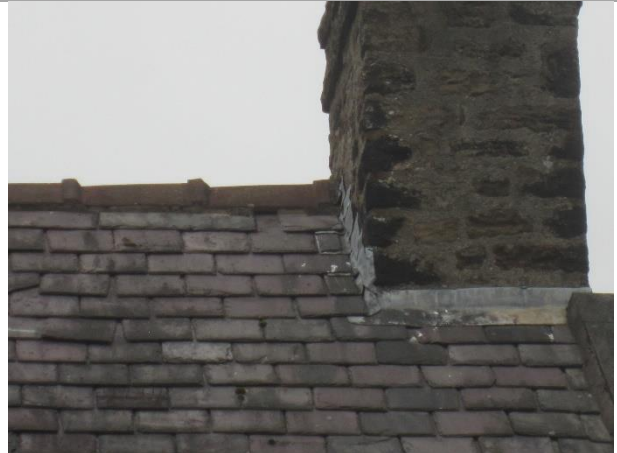
Photo 12: Gaps at ridge copings at farmhouse
