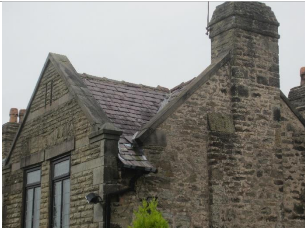
Photo 9: South-eastern elevation showing gaps into roof void
