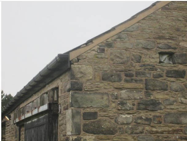
Photo 21: Gaps in stone work and roof verge at Barn A
