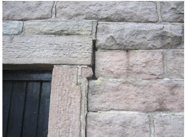
Photo 22: Gaps in stonework at Barn A
