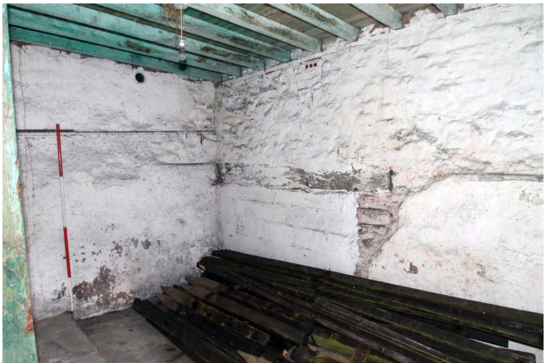
Plate 15. Barn, room G1, south west end, showing blocked doorway, viewed from east.
