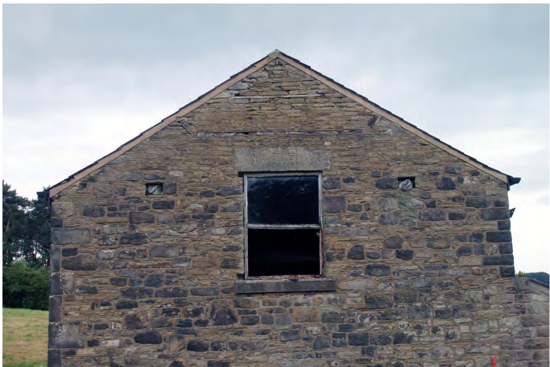
Plate 9. Pike of barn east elevation, viewed from east, showing ex situ datestone over window.
