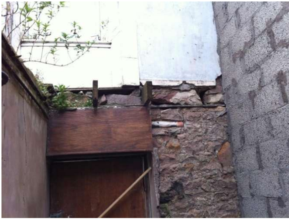
Unsupported, dangerous, condition of walling
