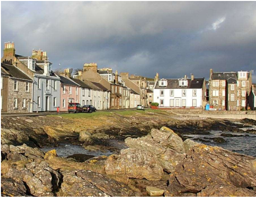
Historical View – the roof to the property is no longer in place.
