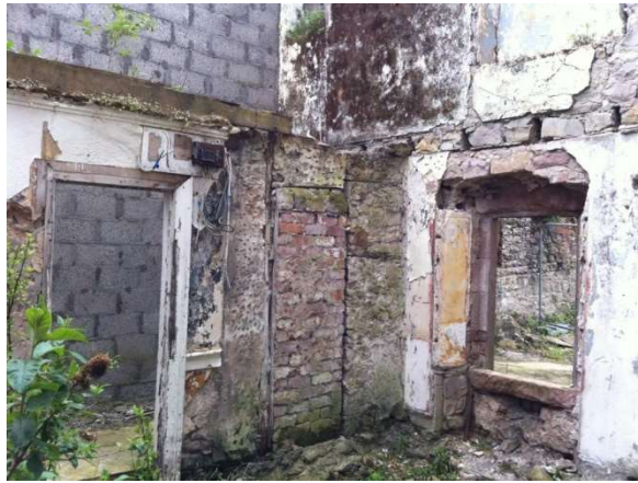
Unsupported condition of internal walling
