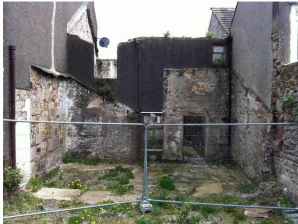
No roofs remain to the property
