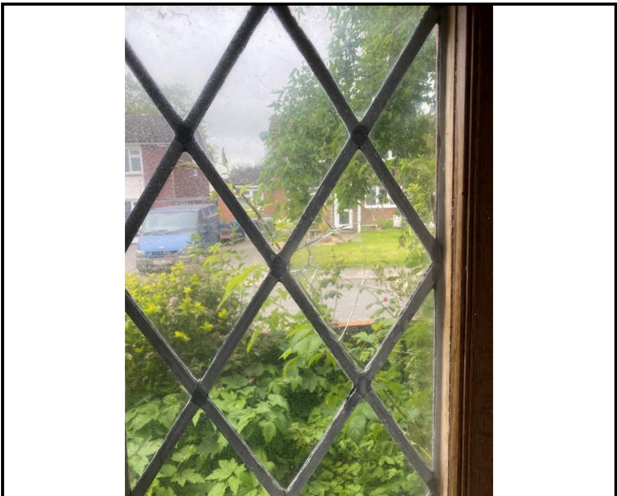
PHOTO 10 – Criminal damage to ground floor window on principal elevation
