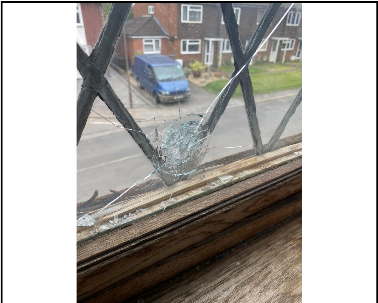
PHOTO 8 – Criminal damage to first floor window on principal elevation
