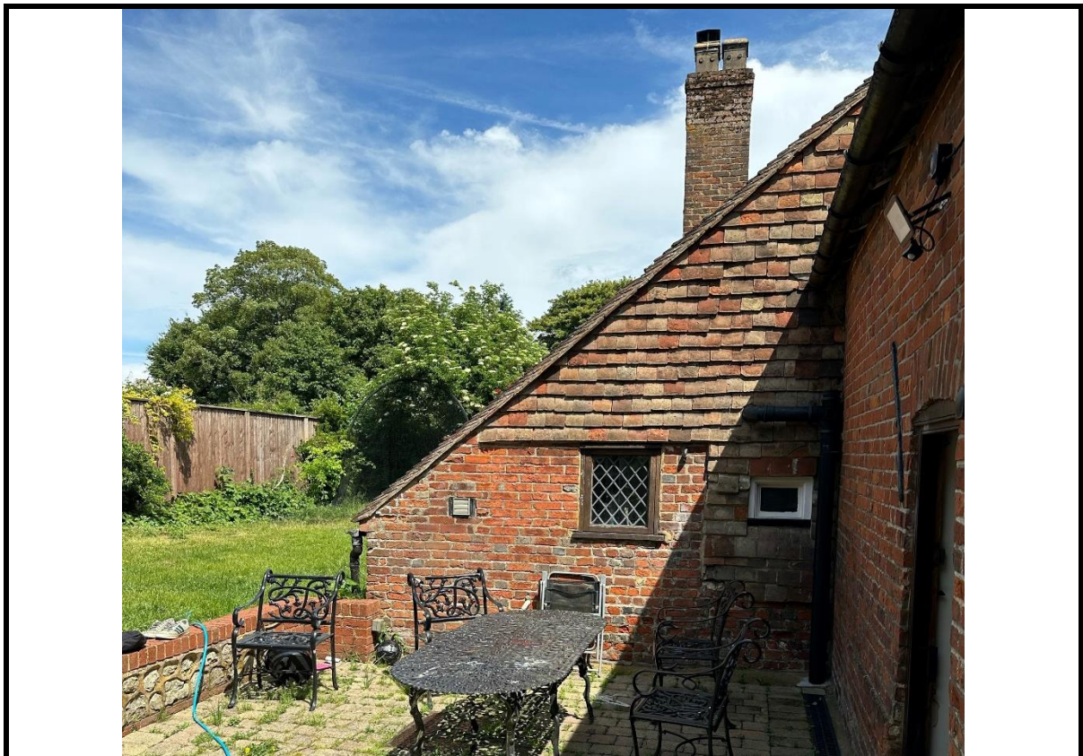
PHOTO 4 – Rear (North) Elevation 1no. window to be replaced.
