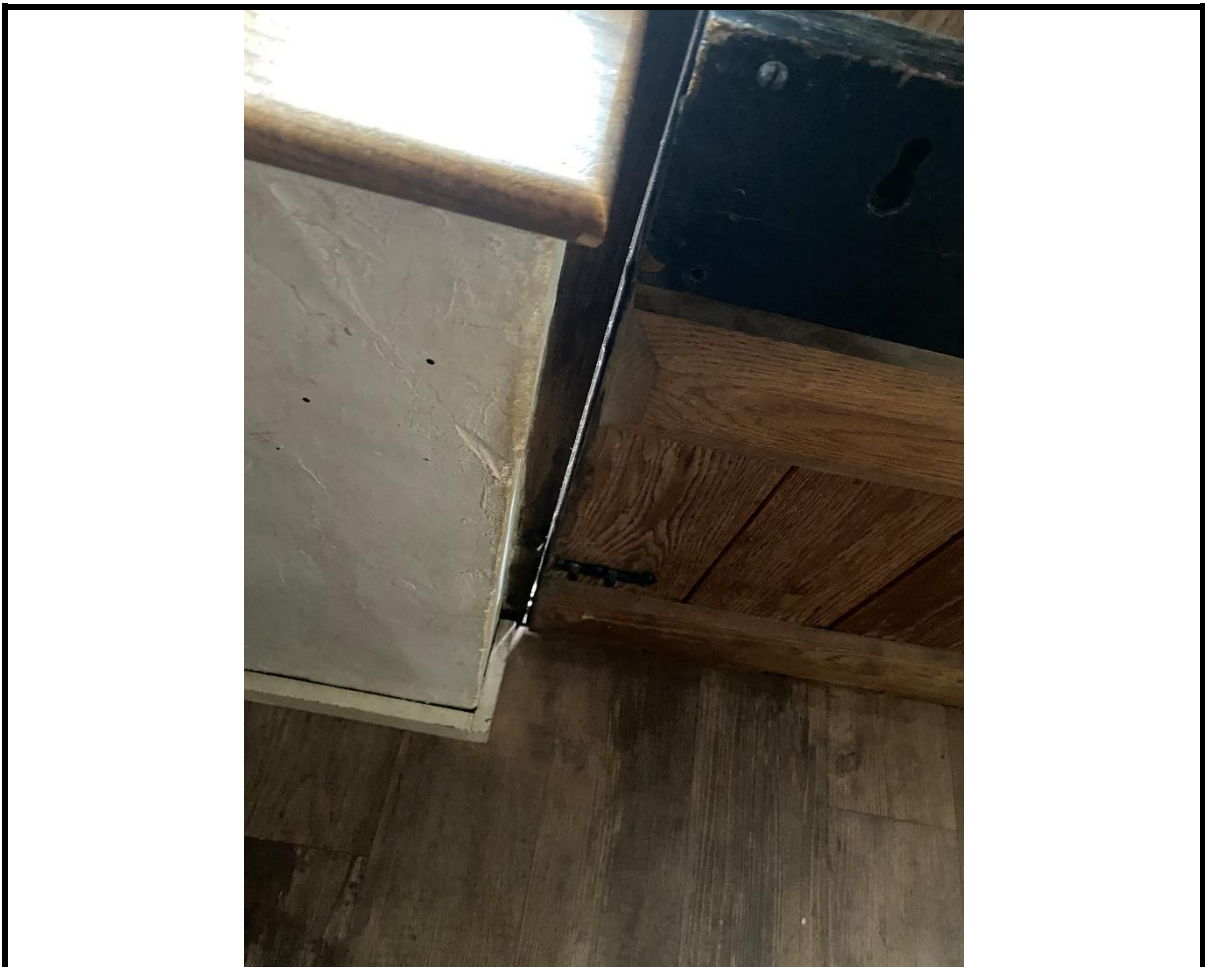
PHOTO 6 – Evidence of warped front door no longer closing properly.
