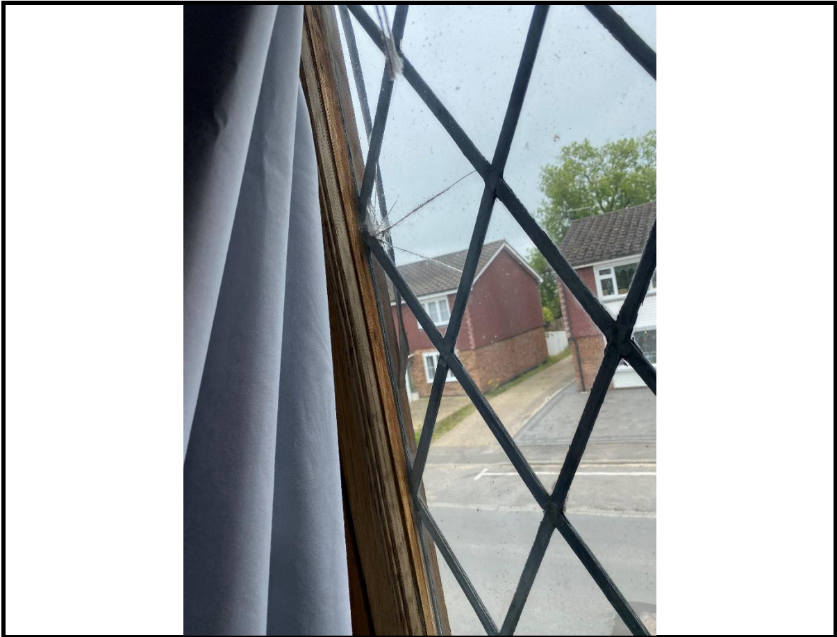
PHOTO 9 – Criminal damage to first floor window on principal elevation
