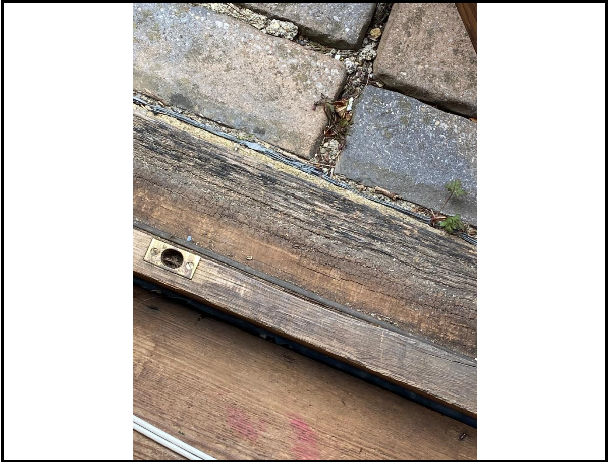
PHOTO 7 – Side door decay and warping causing issues closing.
