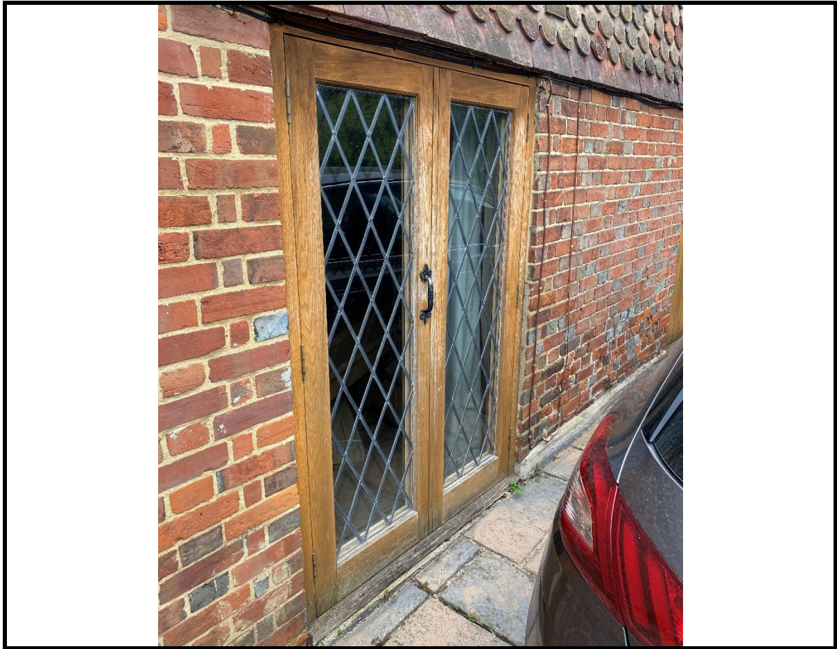
PHOTO 3 – Side door to be replaced on Eastern Elevation
