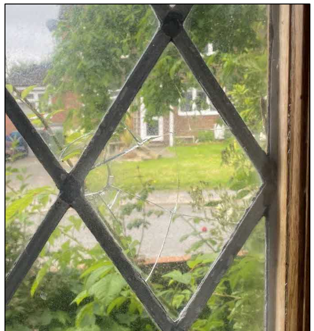
Figure 9 Criminal damage to ground floor window
