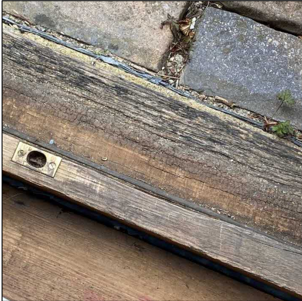
Figure 17: Evidence of rot and warping
