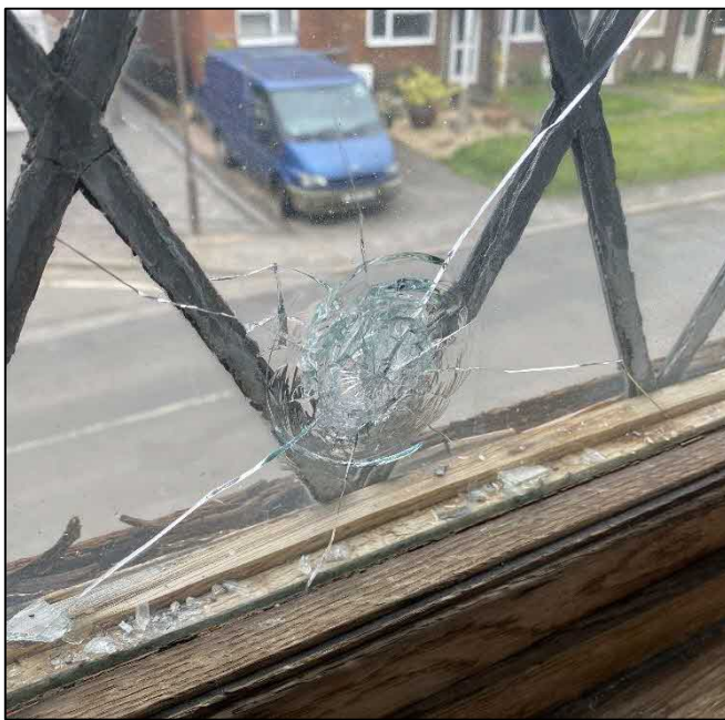
Figure 8: Criminal damage to first floor window
