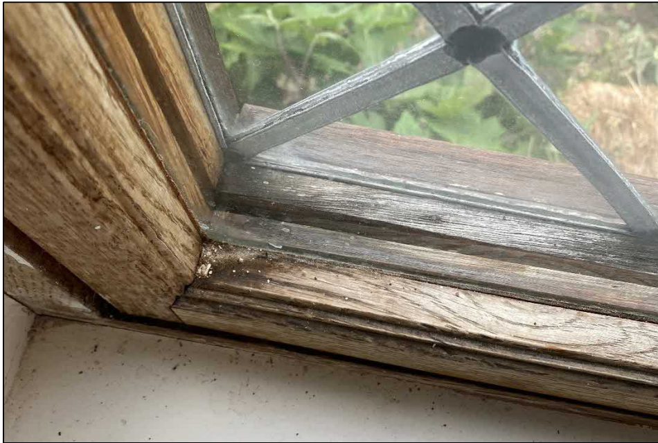
Figure 10: Rotten frame which has separated due to ingress of water and now cannot be opened.
