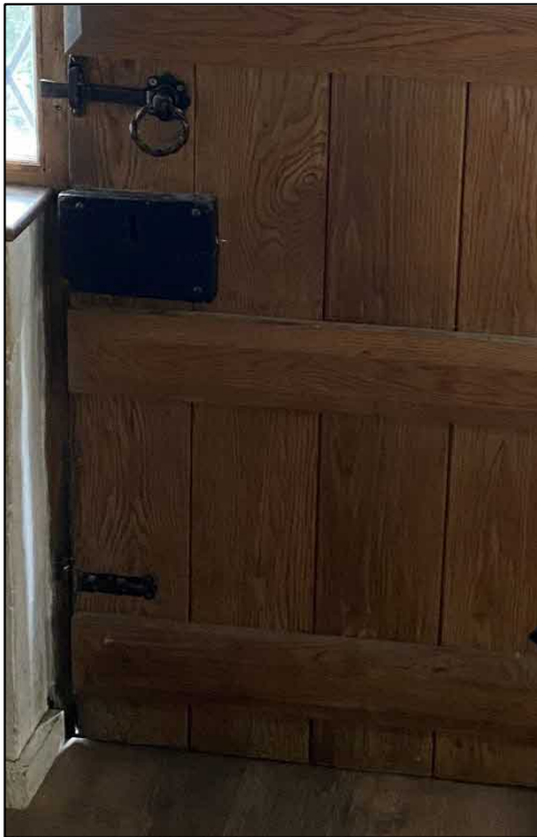
Figure 15: Evidence of front door warping
