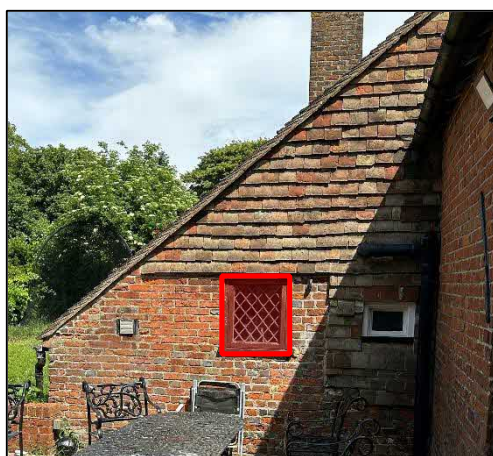
Figure 4: Window to be replaced on the rear elevation.
