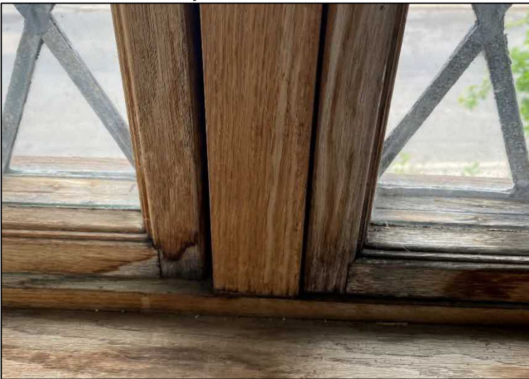
Figure 12: Evidence of condensation and rot.
