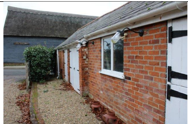
Two A-series light bulbs encased in glass on northern outbuilding, western elevation.
