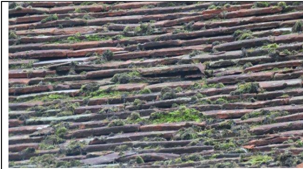
Lifted pig tiles on Church Close House
