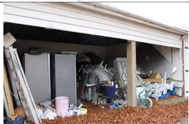
Open-fronted mid-section of northern outbuilding with stored items and a layer of fallen leaves
