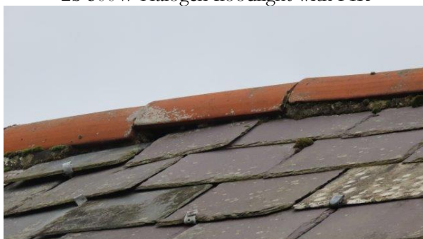
2c Lifted ridge tiles with missing mortar
