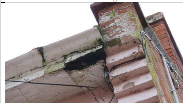
Hole in rotten soffit board on Church Close House, northern elevation
