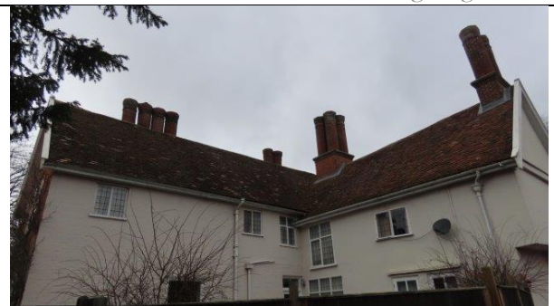
Southern elevation of Church Close House and eastern elevation of southern dormer.
