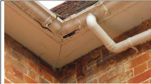
Hole between guttering and soffit on concave corner of the southern extension's western elevation.
