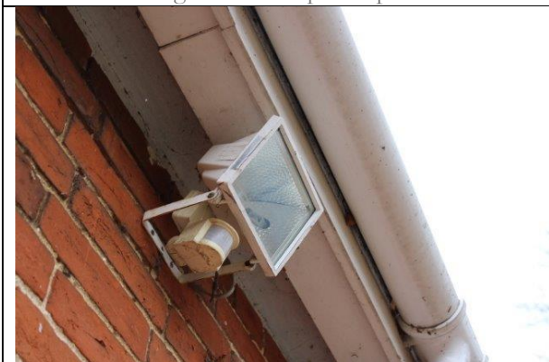
500W halogen floodlight with PIR
