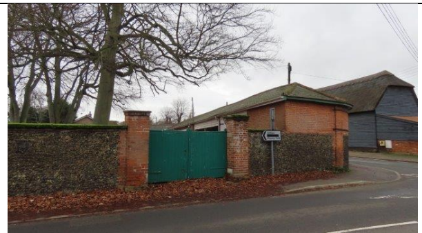
Flintstone and brick walls on north-east border of site. Small gaps under double gate provides potential access points to hedgehogs.
