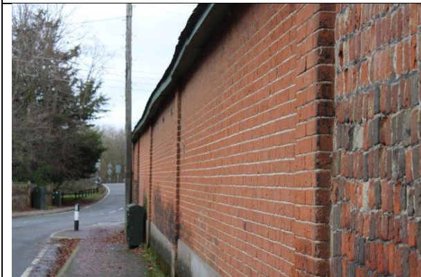
North elevation of northern outbuilding, directly bordering a road and public pavement.
