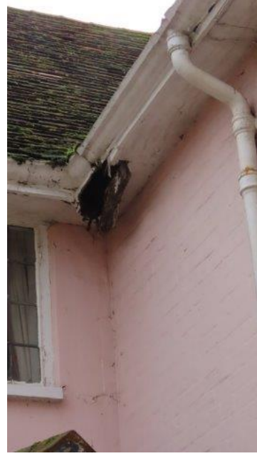
Torn soffit boarding on southern elevation- western end
