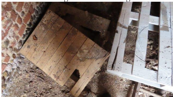
2d Wooden pallets in western section, covered in cobwebs and several rodent and bat droppings
