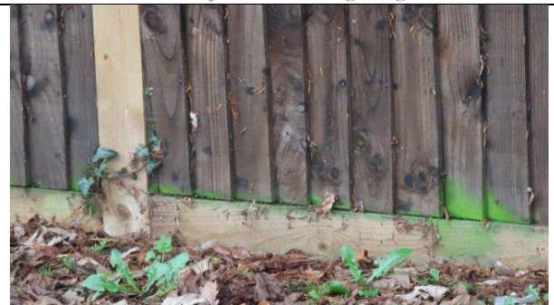
Timber panel fencing with gravel boards /baseboards filled gaps beneath the fencing, and acted as a barrier to terrestrial animals, such as hedgehogs.
