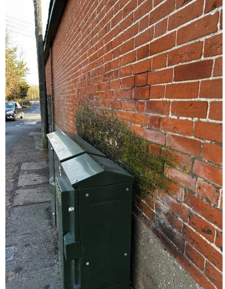
Generally, the wall has suffered from the transfer of water from the highway along with general traffic. As a result, the mortar joints and a number of bricks are worn. A render plinth has been installed at low level.
