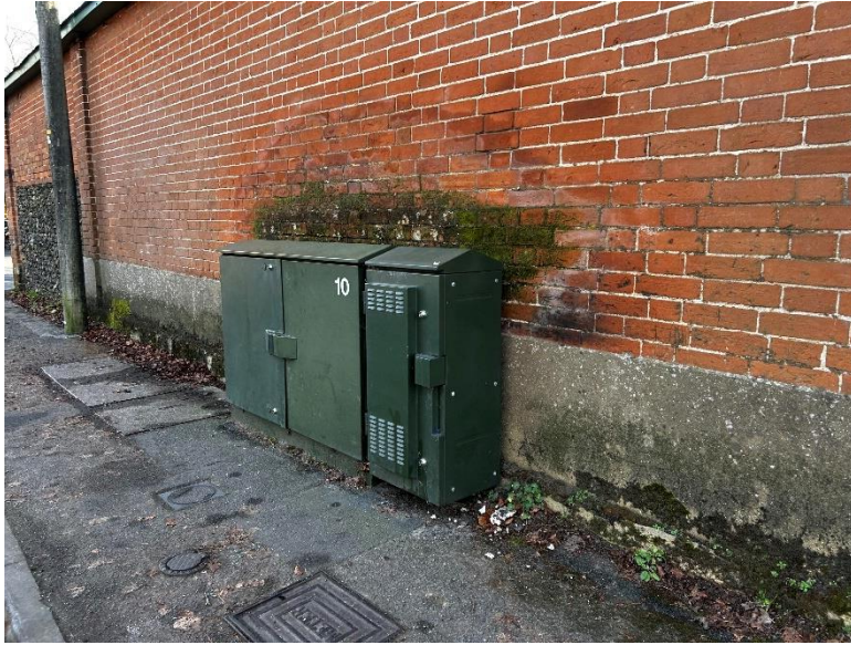
A utility cabinet is located adjacent to the wall facing the road. The wall is suffering from extension water damage and moss growth where water transfers from the cabinet.
