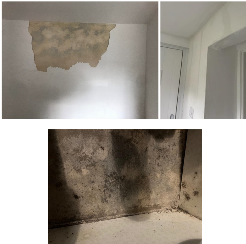
Figures 4 and 5: showing peeling and water ingress that has occurred within a month since re decorating. Figure 6: showing inside kitchen cupboards as example of the black mould throughout the building.
