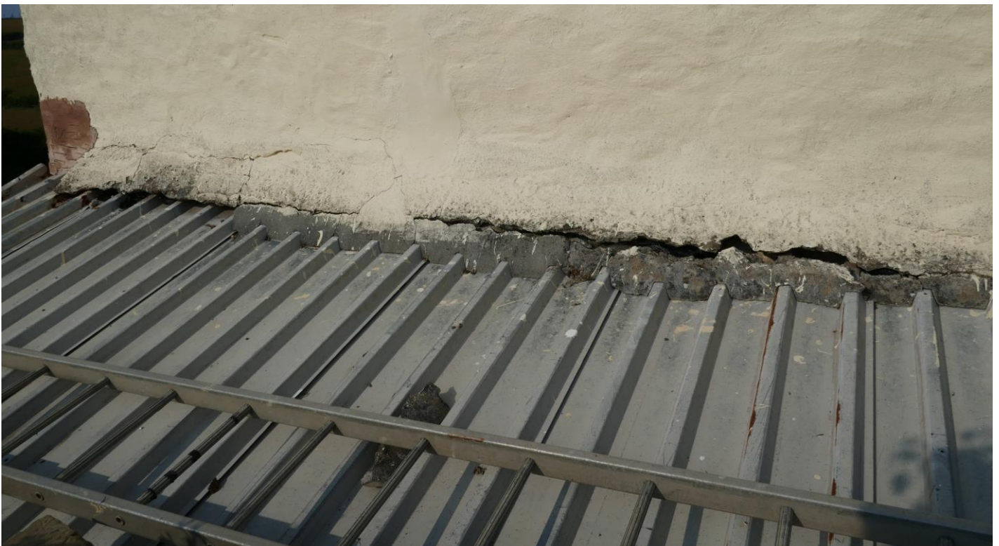
Figure 3. Large gaps at the junction of the house and the lean-to on the western aspect.
