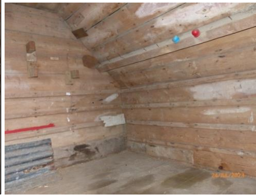
Figure 6: First floor section with wooden panelling beneath clay tiles and behind side panels.
