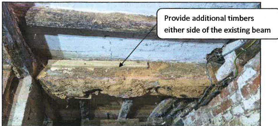
Photograph 3: Rotten timber floor beam
